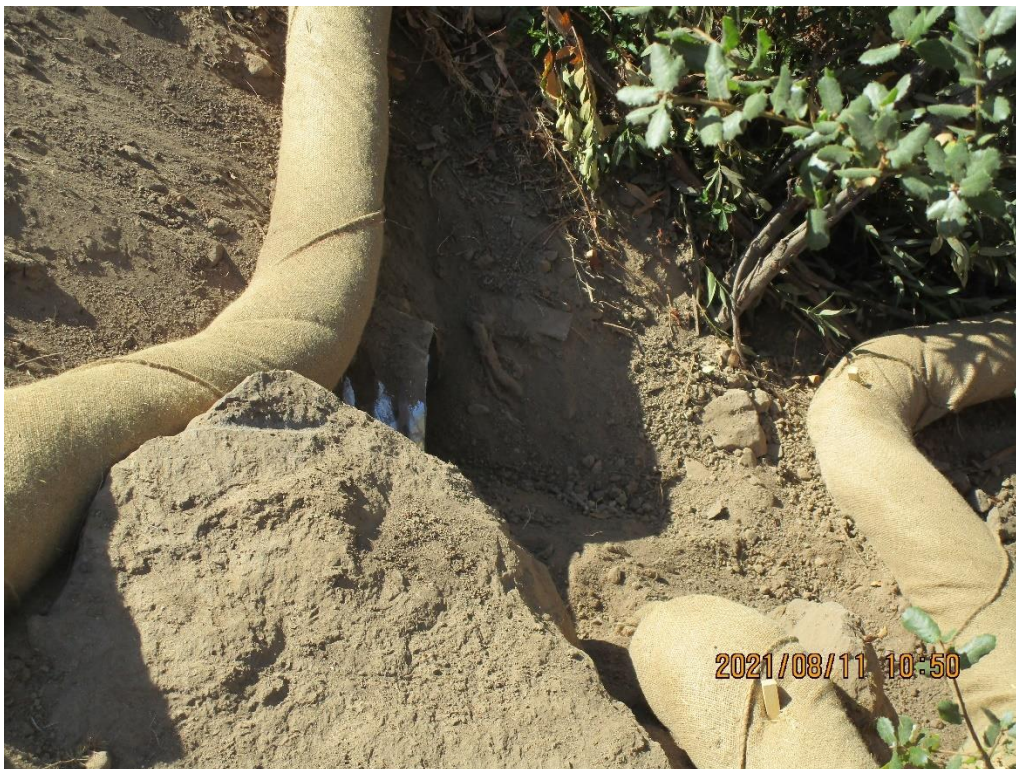
Photo 2. Outlet of new unauthorized culvert, wattles, and fine sediment at WQ5.
