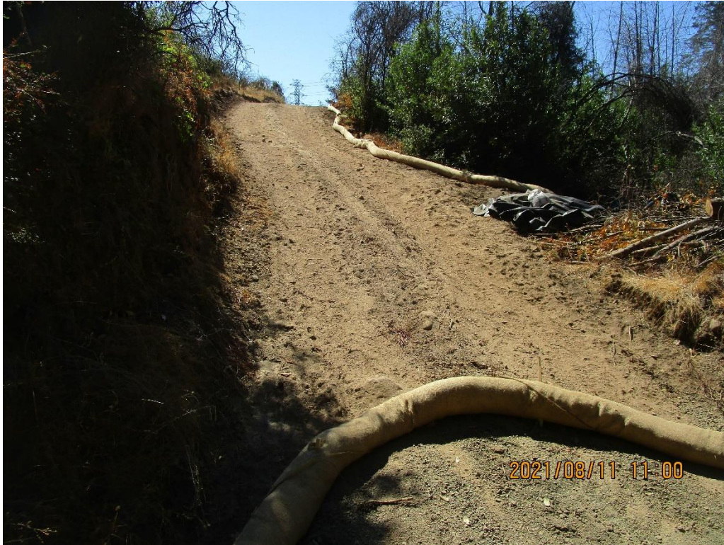
Photo 1. Road segment south of WQ5 with representative example of straw wattle installation.
