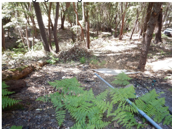
Photo 6: View of the greywater pipe discharging to the ground.
