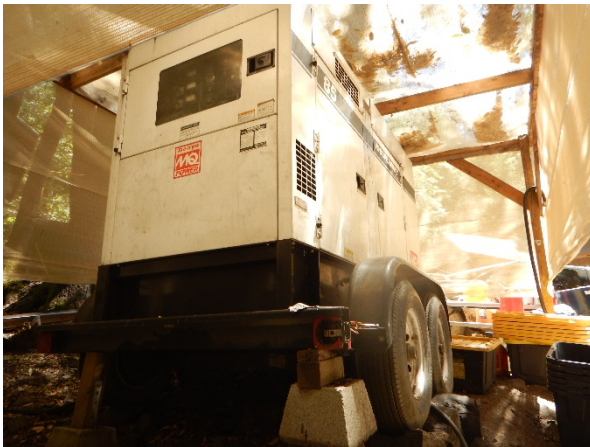
Photo 3: A large mobile generator located near the residence.
