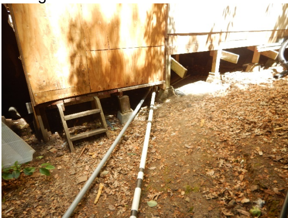
Photo 5: View of the greywater pipe exiting the residence.
