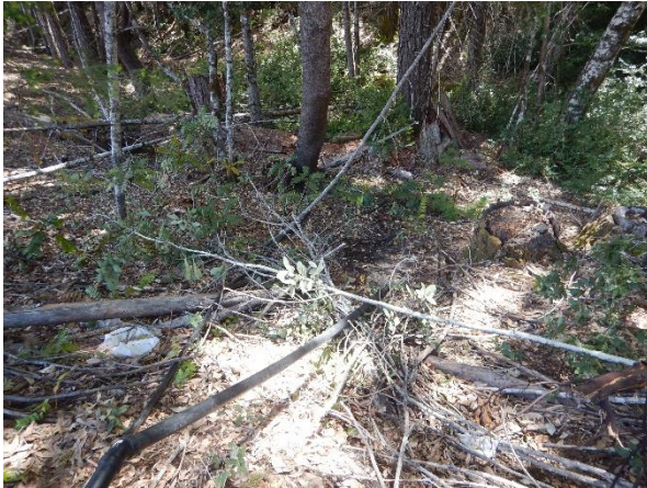
Photo 7: View of the greywater pipe near the Class II watercourse.
