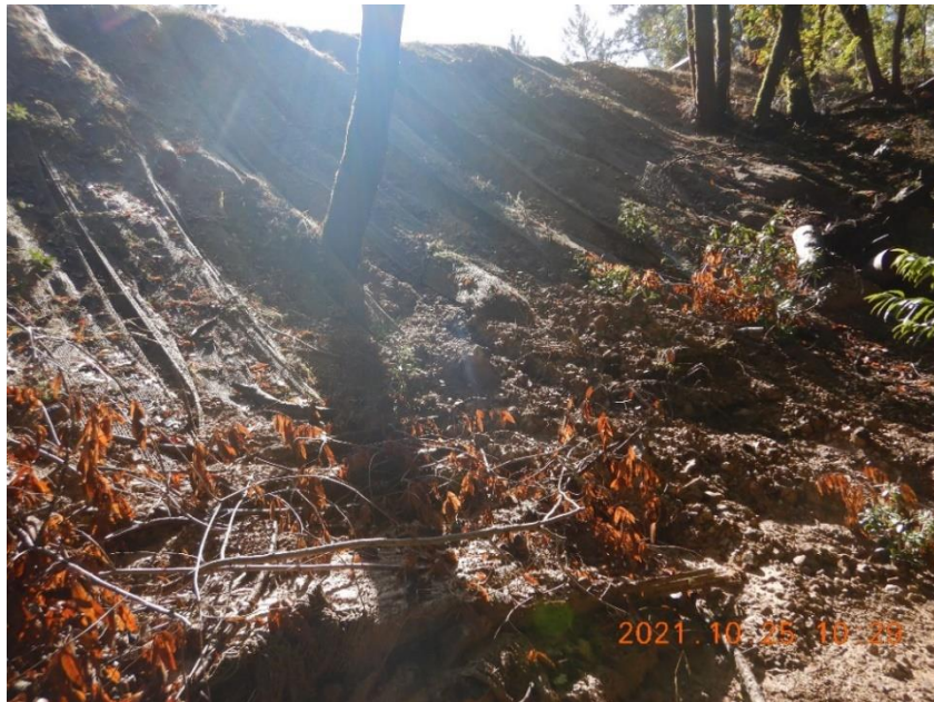
Photo 12—Looking South at western edge of graded pad in the vicinity of WQ8. Gullies are visible below jute netting along the steep fill face. Staff measured one of the gullies to be 42 inches deep with a tape measure. Using a conservative estimates of 18 inches for the average gully widths, 3 feet for average gully depths, 20 feet for average gully lengths and a spacing interval of one gully every 3 feet over 100 feet of gullied fill face visible in aerial images, an estimated 3,000 cubic feet of fine sediment had evacuated from the fill face along the western edge of the constructed pad.
