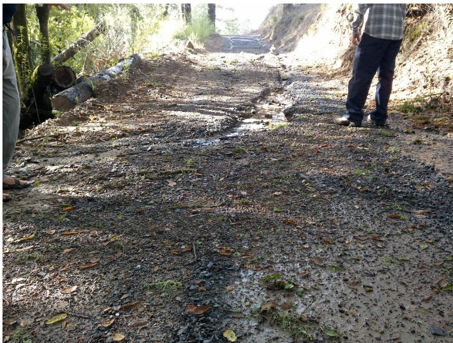
Photo 5—Looking south at WQ4 where stormwater has concentrated on and scoured into the road surface. A berm and woody debris border the downslope side of the road (left side of the image).
