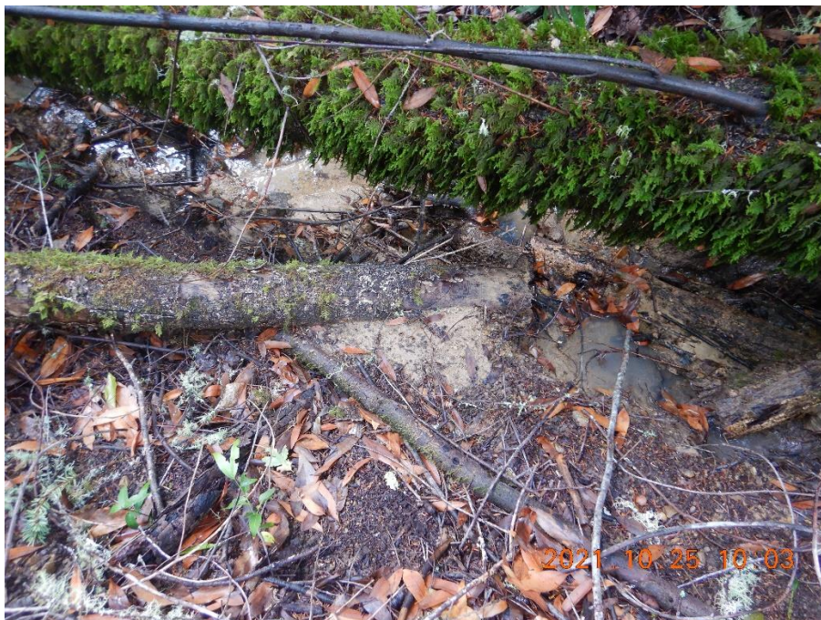
Photo 9—Watercourse, with flowing water, approximately two feet wide at WQ6. Lobes of fine sediment are visible obstructing the flow in the middle of the image.
