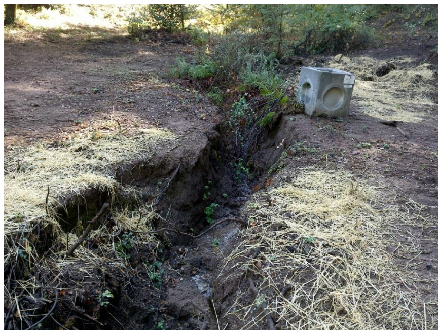
Photo 20—Looking south and upslope at a recently excavated trench within a watercourse. The trench is two feet wide and four feet deep. A concrete cube (drop culvert inlet) is next to the excavated channel. Staff advised Mr. Vattuone that a WDR from the Regional Water Board is required prior to excavating material from a stream channel.
