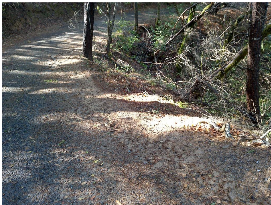
Photo 4—Looking south along road in the vicinity of WQ3. Stormwater has scoured the road surface where a low berm on the downslope side of the road (right side of the image) prevents stormwater from flowing off the road.
