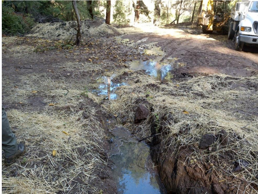
Photo 21—Looking north from excavated watercourse at WQ13. A backhoe and dump truck are visible in the back right of the image. Mr. Vattuone informed staff that he had been excavating sediment from the onstream reservoir to the north and staging it at the proposed culvert locations to use to bury the culverts. Staff advised Mr. Vattuone that a WDR from the Regional Water Board is required prior to dredging material from an onstream reservoir.
