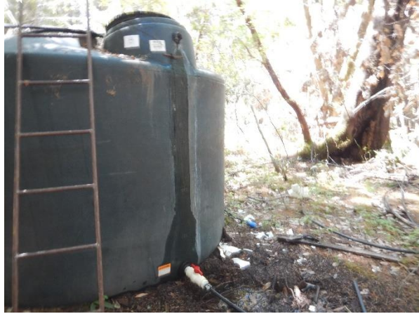
Photo 8: Closer view of TANK1 overflowing adjacent to a Class II.
