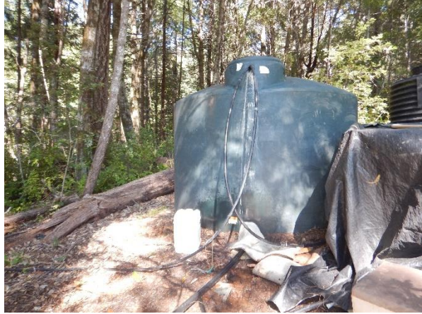
Photo 25: Closer view of TANK2 overflowing near the residence and CA3.
