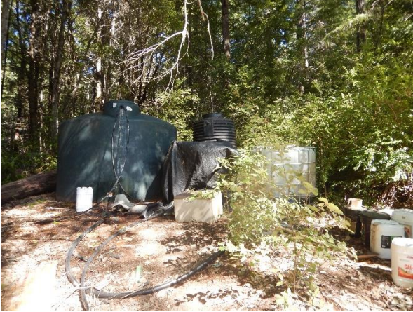
Photo 25: View of TANK2 overflowing with water near the residence and CA3.
