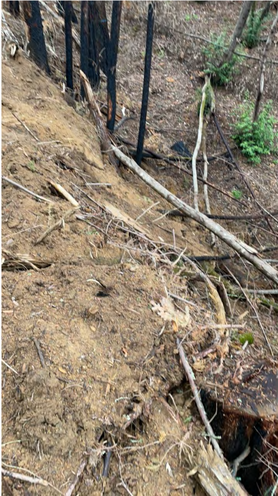
Figure 8. Sidecast material from newly removed waterbars above head of Class III watercourse near Water Quality Map Point 6.
