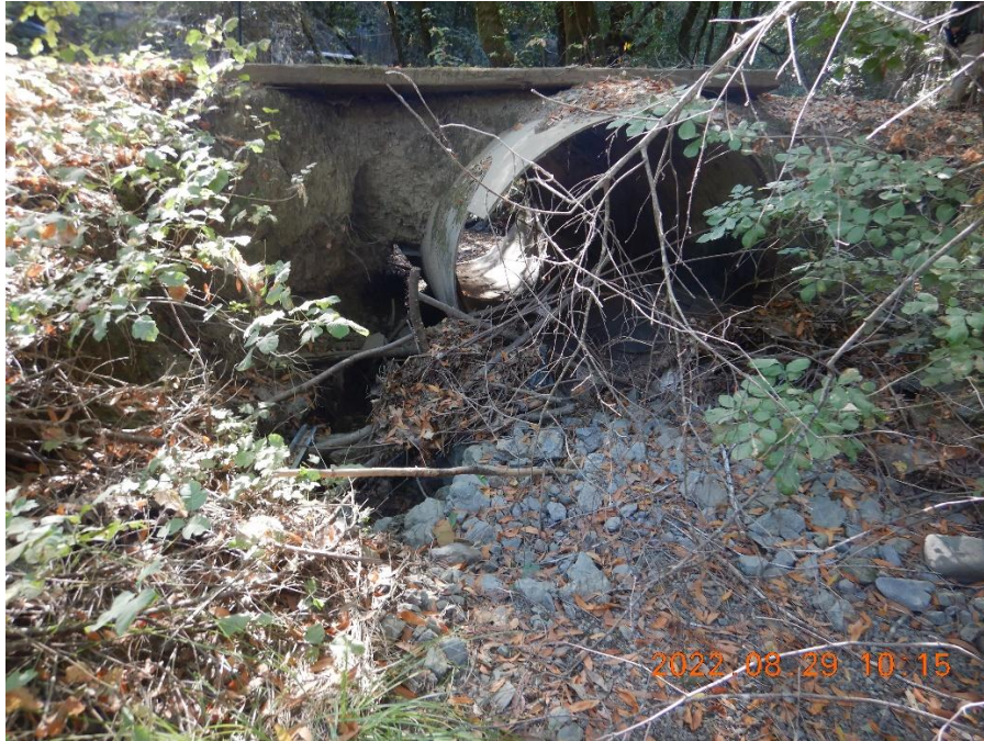
Photo 17—Looking south and downstream at the road crossing Hulbert Creek at WQ9. Debris is visible blocking the culvert inlet and a scoured channel appears to the left of the culvert.
