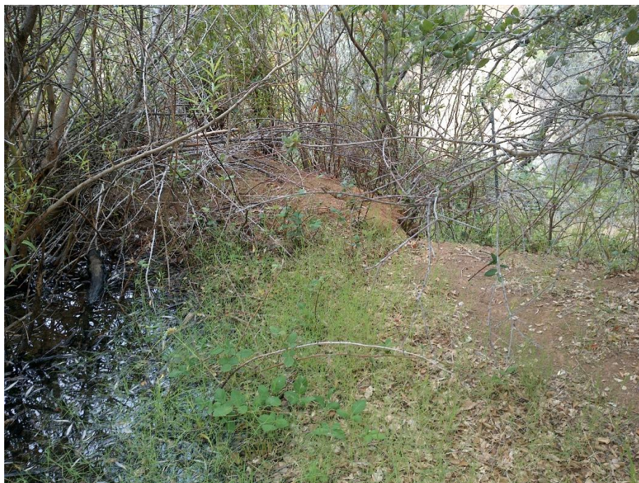
Photo 8—Berm on western side of reservoir located at WQ3. The berm is only 2 feet wide at the narrowest point.
