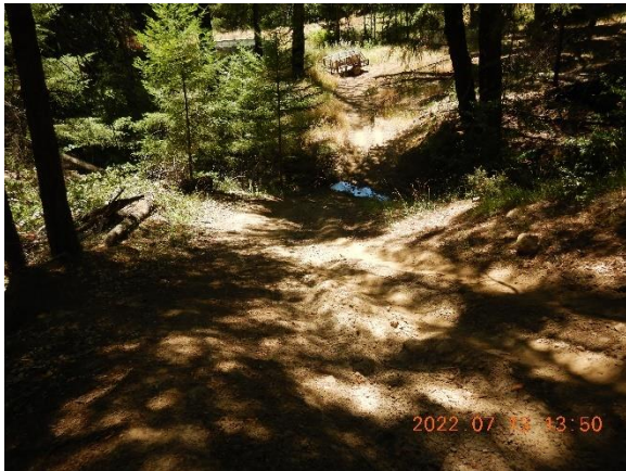
Figure 24. WQ5, WP803. Stream Crossing 2 is a wet ford on a Class II watercourse, with direct delivery from the road surface.
