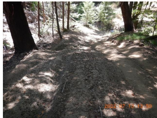
Figure 23. WQ5, WP803. Upslope of Stream Crossing 2, the steep rutted road surface is hydrologically connected to the stream crossing for 170 feet.
