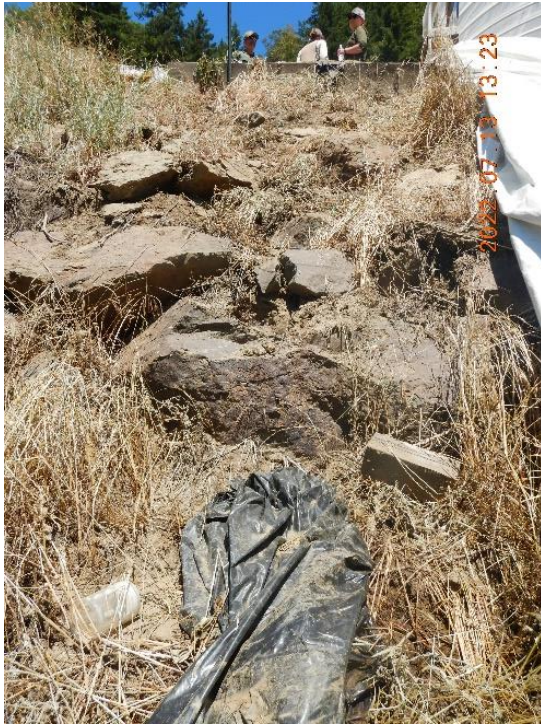
Figure 15. Rock on fillslope upslope of culvert outlet.
