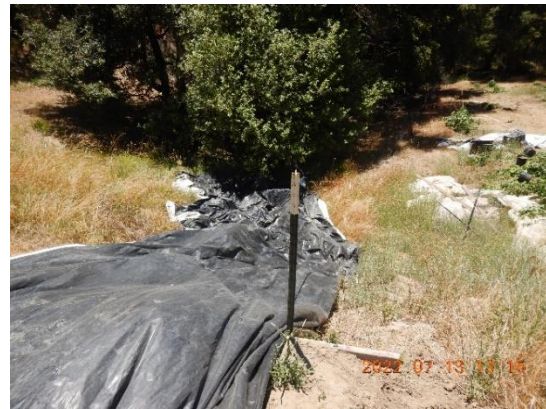
Figure 14. WQ2. WP795. A corrugated plastic pipe protrudes from fill slope associated with constructed flat used for cultivation (CA3). Photo shows plastic sheeting over the culvert outlet and fillslope, down to watercourse channel.
