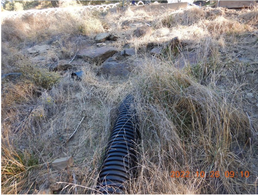
Figure 12—Corrugated plastic pipe located at WQ2. Aerial imagery shown in Figures 2 through 5 above suggests the pad in the background of the image buries a surface watercourse.
