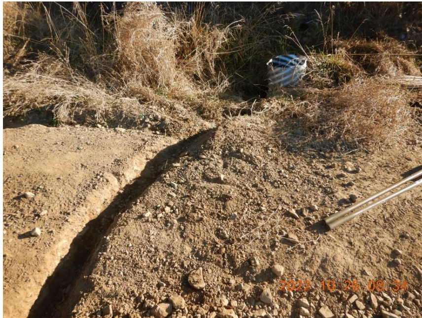
Figure 10—Looking north at culvert inlet located at WQ1. A trench across the road is shaped such that stormwater collected by the road will be directed into the pipe.
