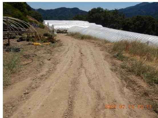
Figure 9. WQ1. CA3 and rilled access road.
