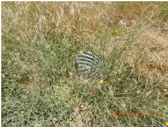
Figure 12. WQ1. Drop inlet upslope of access road to CA3.
