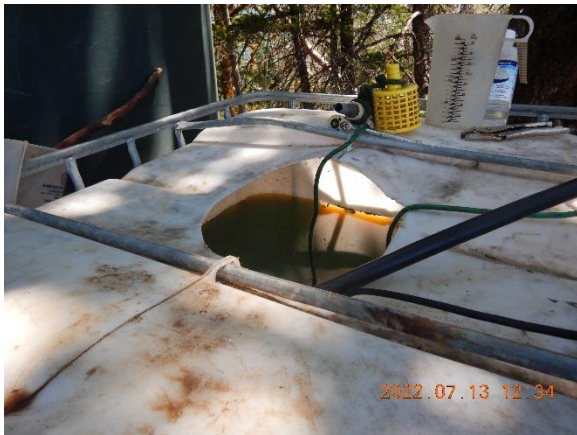
Figure 5. Open top of feed tank at CA1.
