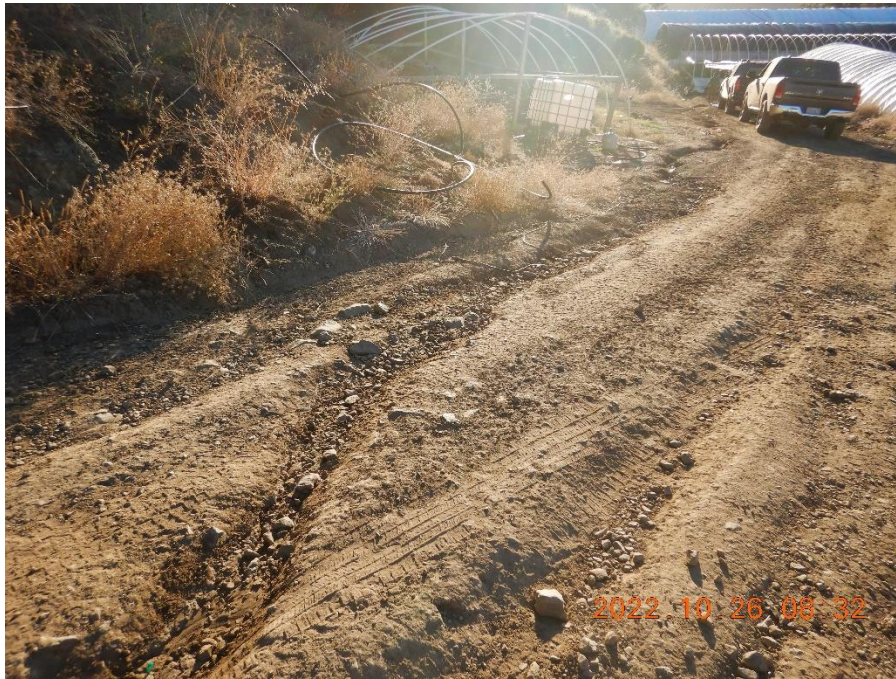
Figure 8—Looking east in the vicinity of WQ1. Wheel ruts on the road surface are visible in the middle of the image.
