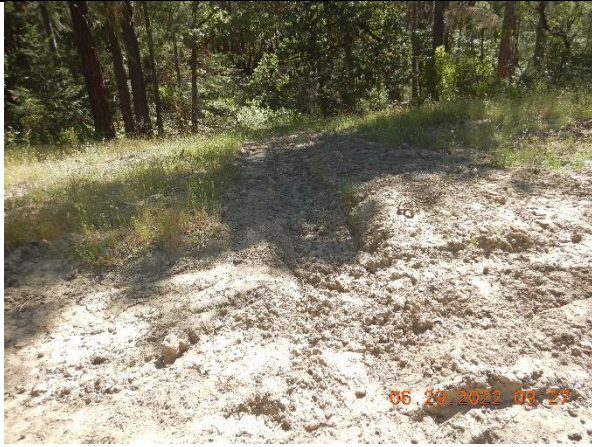
Photo 73: grading within a riparian setback of a watercourse at inspection point WQ10
