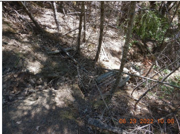
Photo 18: outlet of an improperly installed culverted stream crossing at inspection point WQ13
