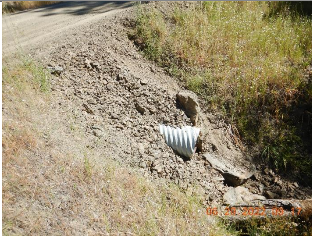
Photo 9: culvert installed high in the fill at inspection point WQ7
