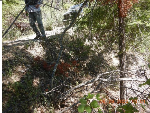
Photo 16: outlet of an improperly installed culverted stream crossing at inspection point WQ12
