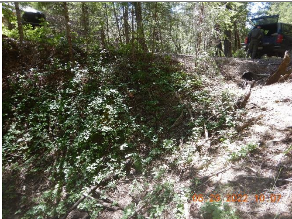
Photo 17: inlet of an improperly installed culverted stream crossing at inspection point WQ13
