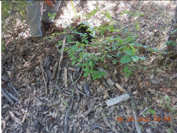
Photo 15: inlet of a culverted stream crossing installed high in the fill at inspection point WQ12
