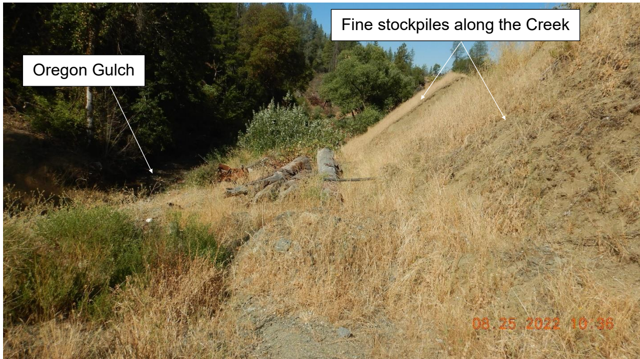
Photo 3: Looking southwest at naturally vegetated fine materials stored adjacent to Oregon Gulch. Potential discharge point. Picture taken by Farzad Kasmaei.
