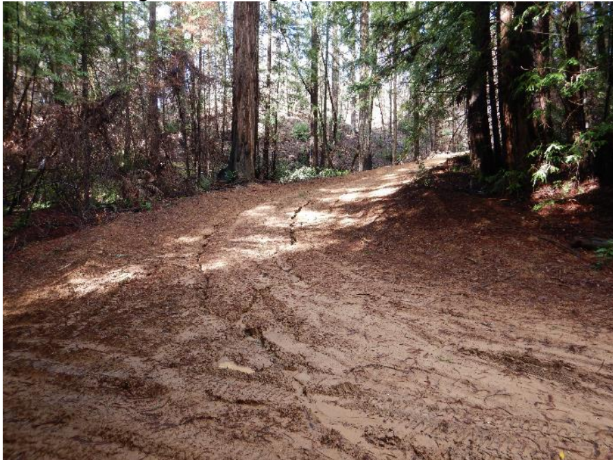
Photo Point 2.1 - Road segment, looking uphill. 11/04/2021
