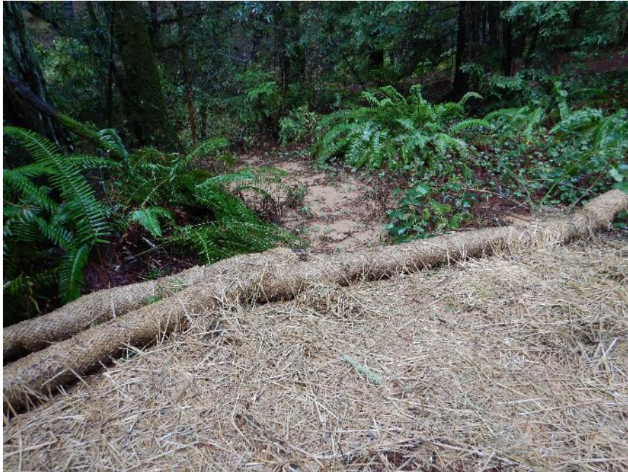
Photo Point 2.6 - Erosion control measures at base of hill, on banks of Felta Creek, installed after storm of October 24, 2021. 11/04/2021
