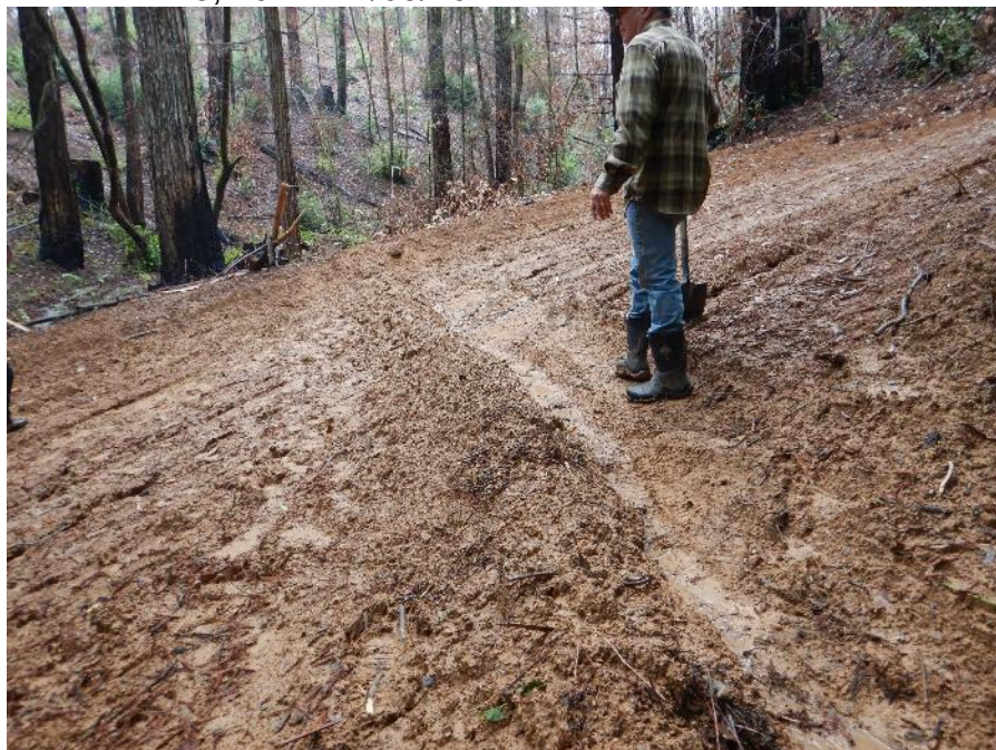
Photo Point 2.7 - Waterbar, newly installed between inspection of November 4, 2021 and rains of November 8, 2021. 11/08/2021
