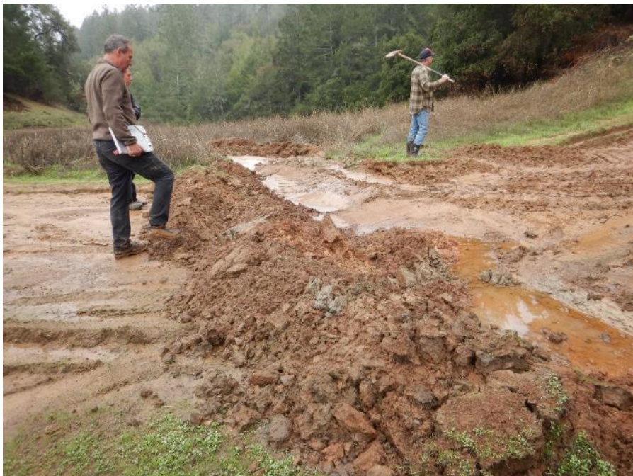
Photo Point 4.3 – Newly installed waterbar on haul road. Installed during saturated soil conditions. 11/09/2021
