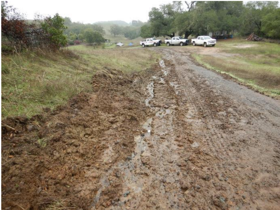
Photo Point 4.1 – Rilling on haul road downhill of newly installed waterbar. 11/09/2021
