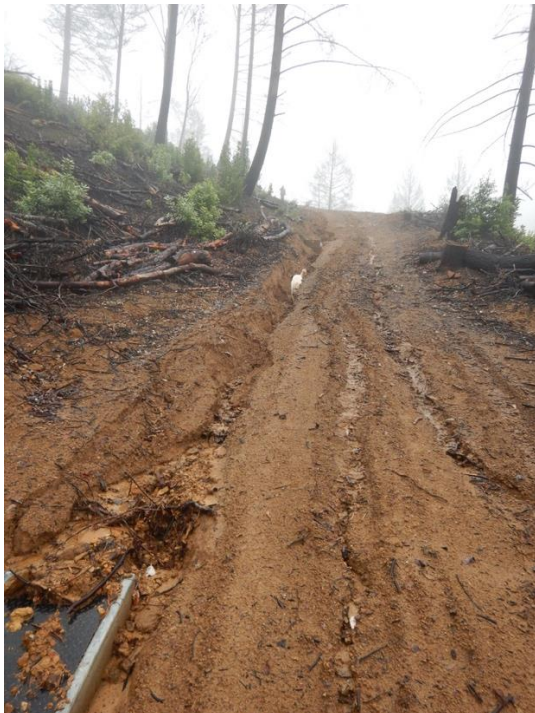
Photograph 3. The photograph shows rilling and gulying of road surface. What appears to be a remnant rolling dip is present near the top of the road.
