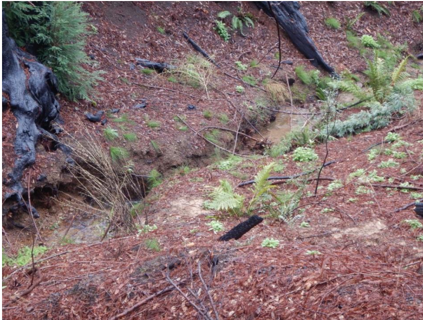
Photograph 4. The photo shows road material entrained in redwood duff immediately adjacent to an unnamed perennial tributary to Mill Creek. Road material is also visible within the watercourse channel.
