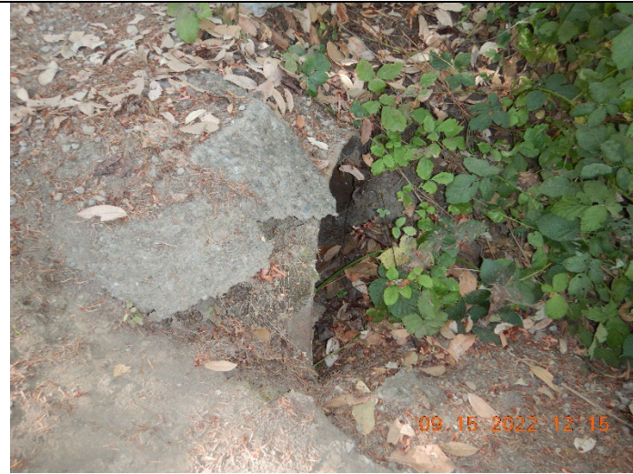
Photo 1: Partially clogged outlet of a culverted stream crossing at inspection point WQ1
