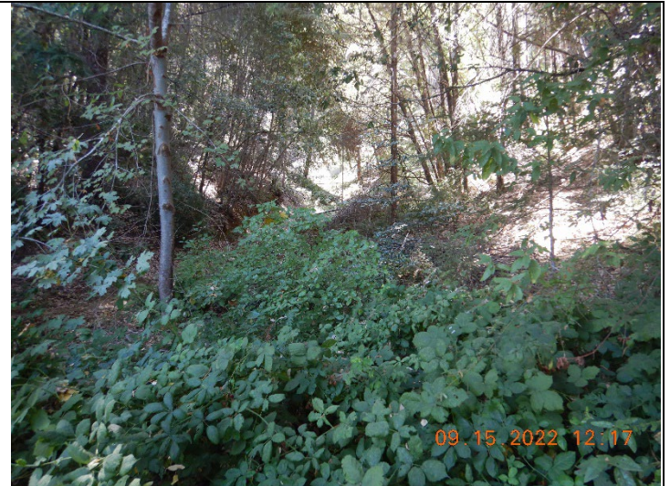
Photo 2: vegetated stream channel at the inlet of a partially clogged stream crossing at inspection point WQ1
