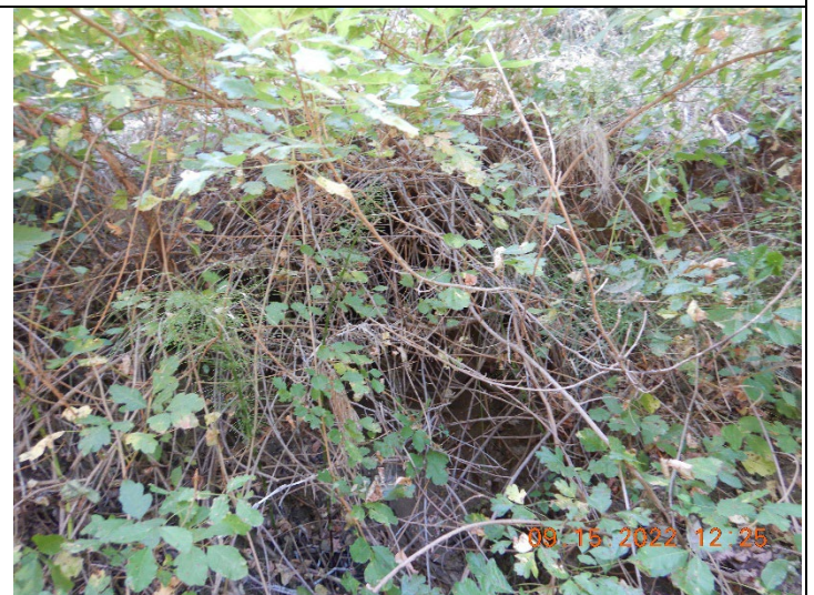
Photo 4: Outlet of a culverted crossing covered with vegetation at inspection point WQ2
