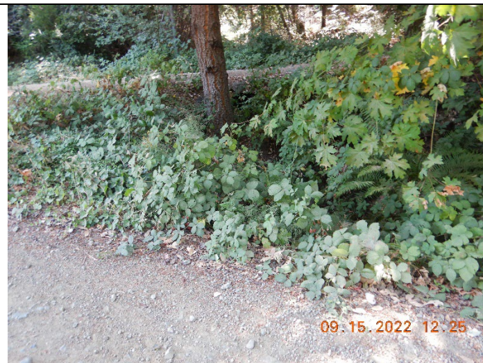
Photo 3: Vegetation covered inlet of a culverted stream crossing at inspection point WQ2
