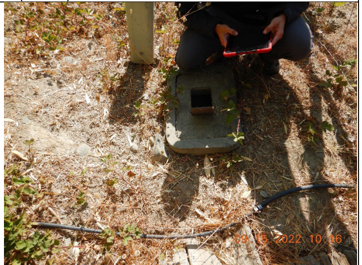
Photo 4: Municipal water source meter at inspection point WQ3
