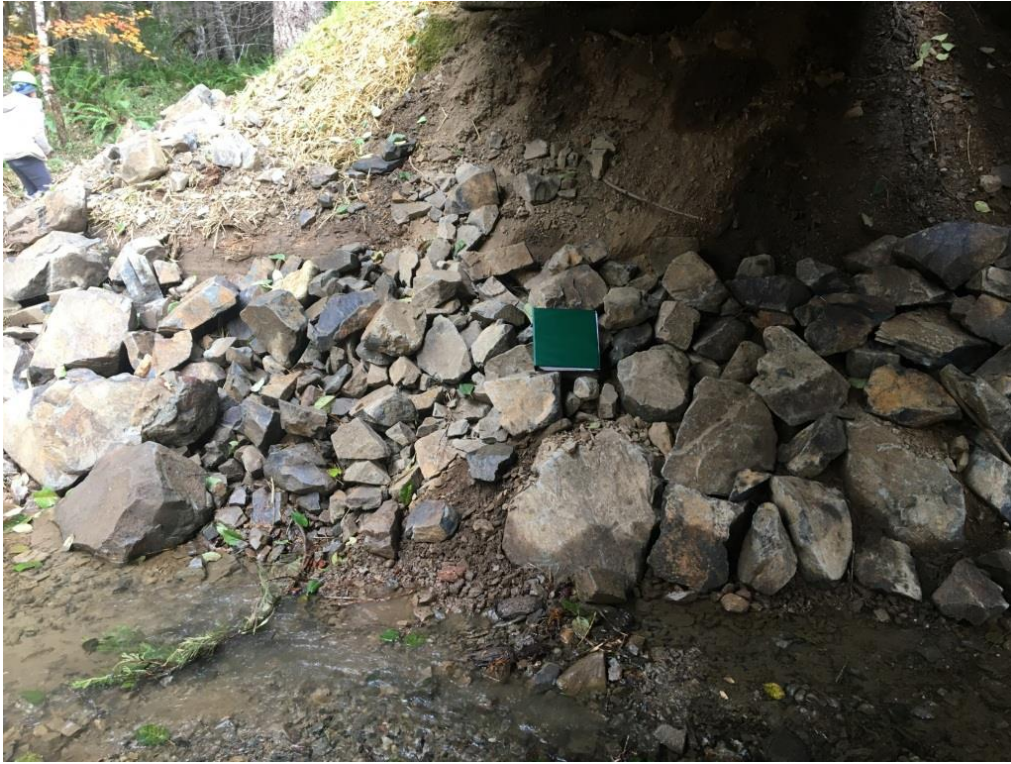
Figure 2. View of RP1 from under bridge facing right bank. Note 1 square foot green binder for scale.
