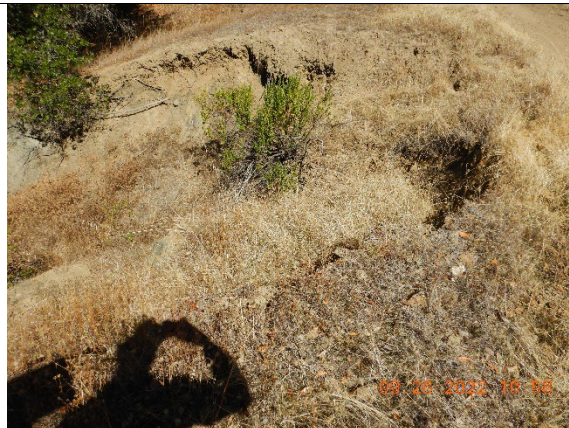
Photo 32 – collapsed roadside fill prism at inspection point WQ20
