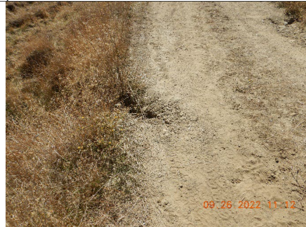
Photo 15 – Road erosion near the inlet of a metal culverted watercourse at inspection point WQ28
