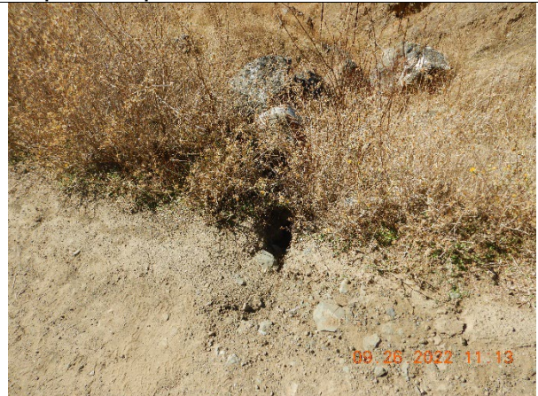
Photo 16 – Road erosion near the outlet at inspection point WQ28
