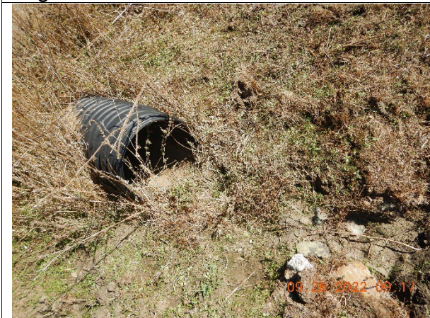
Photo 9 Culvert outlet delivering sediment to surface water at inspection point WQ1
