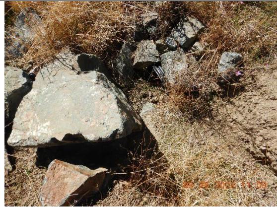
Photo 14 – Plastic culverted watercourse crossing inlet obstructed with rocks at inspection point WQ27
