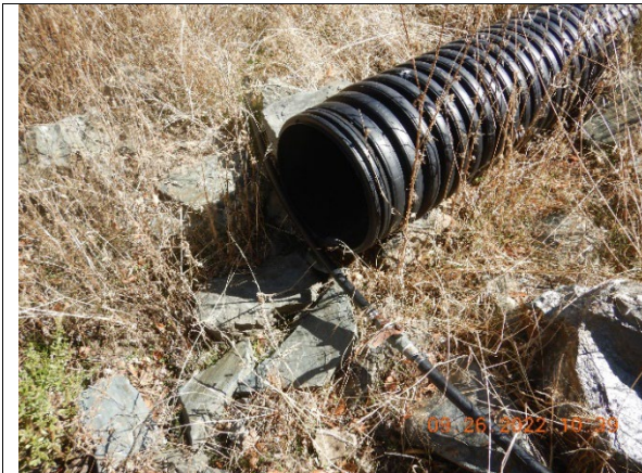
Photo 11 – Properly installed culvert outlet of an onstream pond at inspection point WQ16
