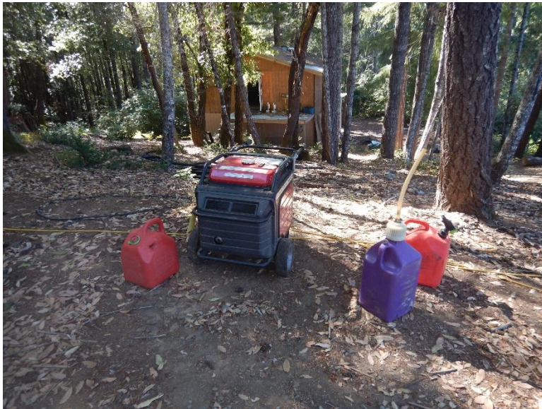
Photo 4: Generator and petroleum products stored outside without cover or containment
