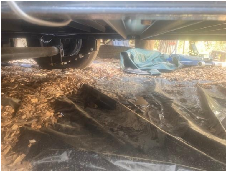
Photo 11 (taken by Helen Bowman): View under generator with inadequate secondary containment and diesel spill evident on tarp.
