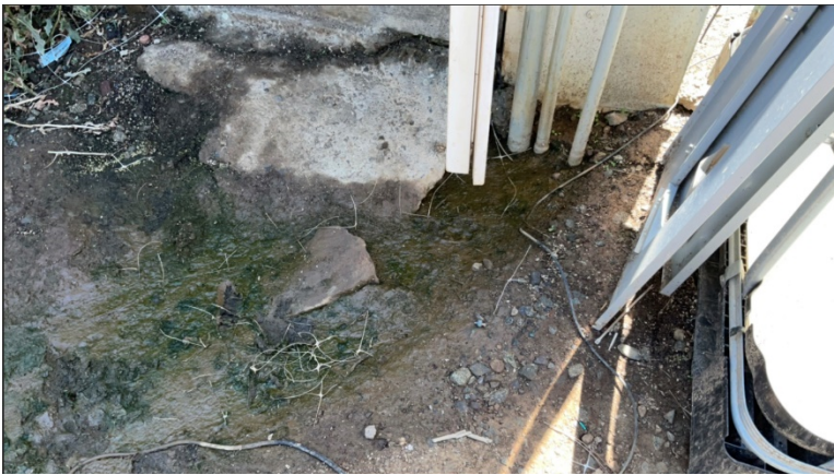
Photo 4: Pipes discharging to ground surrounded by wet soil and algae outside of cultivation building.
