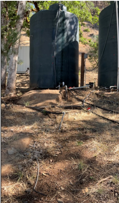
Photo 7: Overflowing water storage tank.
