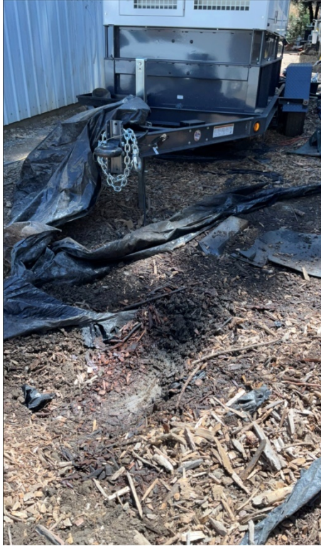
Photo 10: Generator on landing with wood chips and tarps. Black soil concentrated with diesel uncovered. Area smelled strongly of petroleum.
