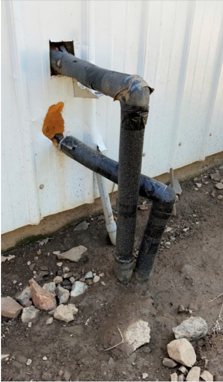
Photo 3: Pipes discharging to ground surrounded by wet soil outside of cultivation building.
