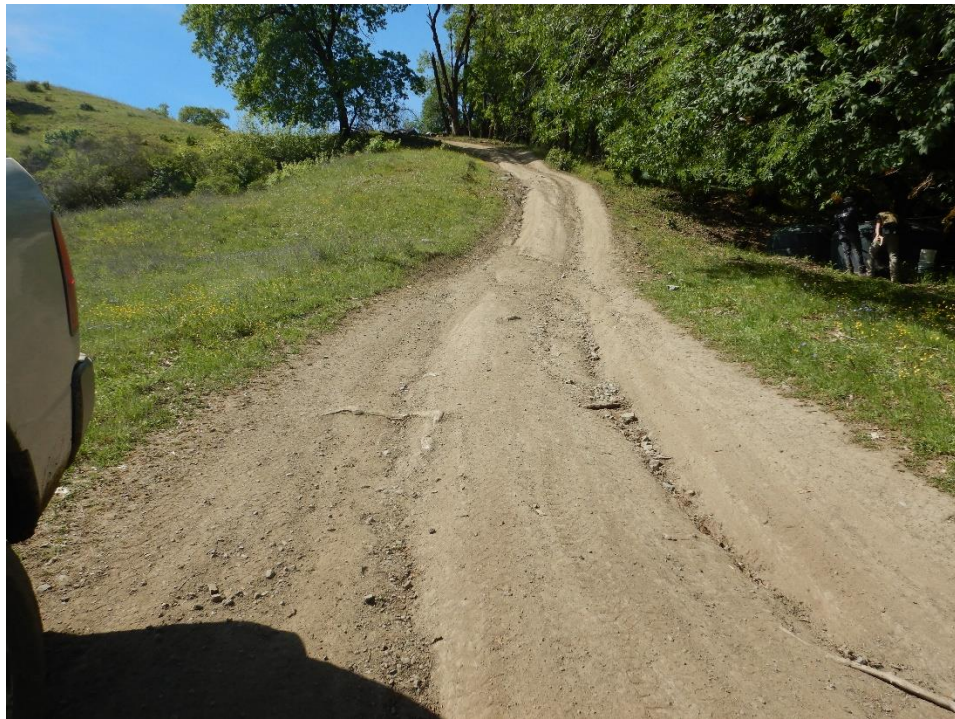
Photo 34—Rutting and rilling on road north of WQ8.
