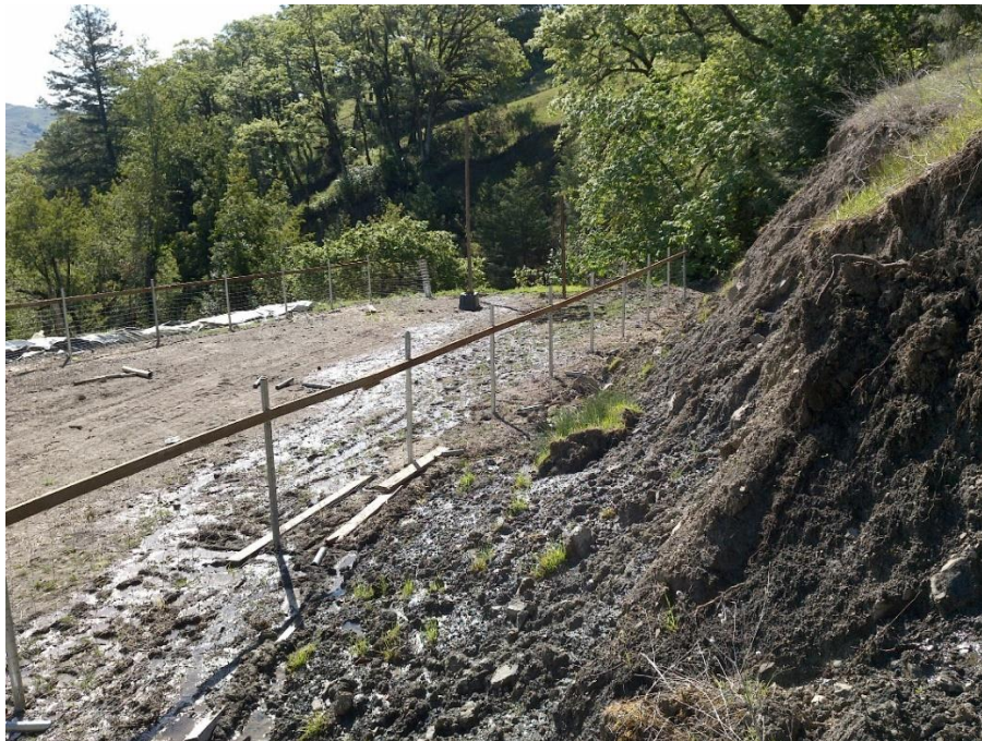
Photo 14— Looking southeast along graded pad south of WQ4. The photographer is standing at the same location as the previous two images. Water emanates from cut-face and flows over cultivation pad to receiving water in the background of the image.
