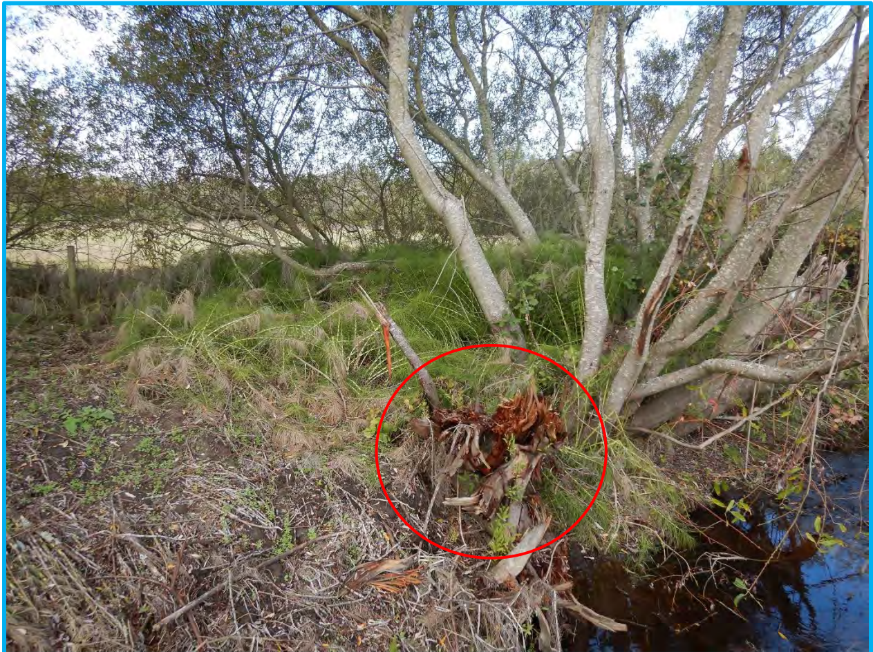
Photograph 7. Photograph of a willow removed by breaking off the trunk (circled in red) using a thumbed excavator. Removal of invasive Himalayan blackberries have occurred on the left-bank leaving native equisetum.
