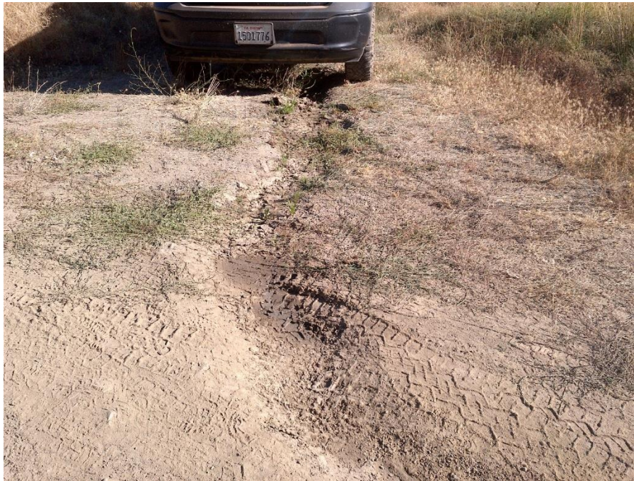
Photo 9—A channel eroded in the road surface by flowing water at WQ4.
