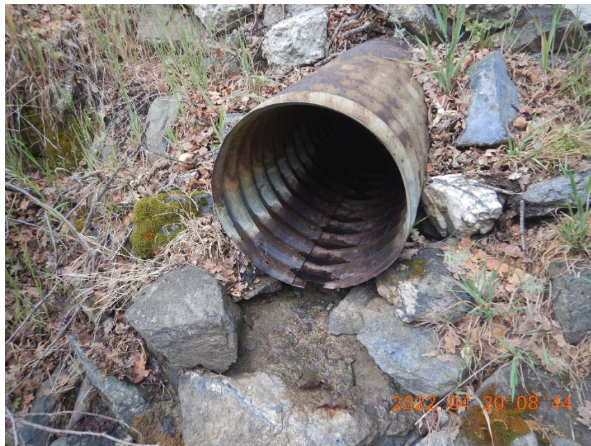
Photo 12— The outlet of the culvert located at WQ6. The pipe is 15 inches in diameter, and 20 feet long. Holes have rusted through the bottom of the metal pipe allowing water to flow below the pipe.
