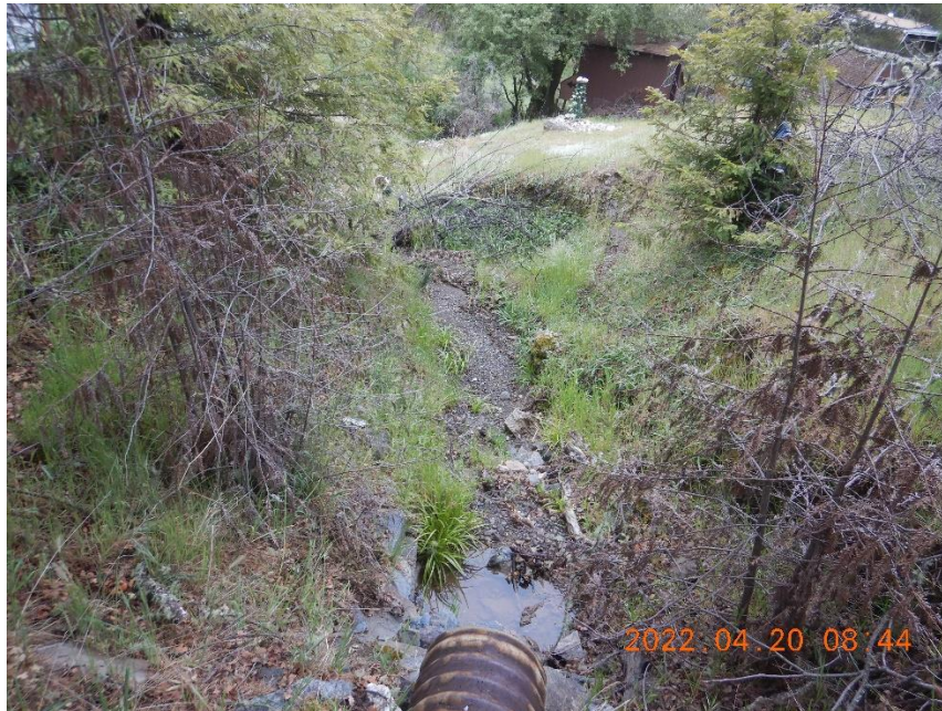
Photo 13— Looking southeast and downstream from the culvert at WQ6. The culvert is perched several feet above the channel bed.
