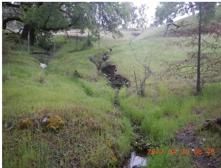
Photo 14— Looking northwest and upstream from the culvert at WQ6. The watercourse width upstream averages between 2 and 3 feet wide.
