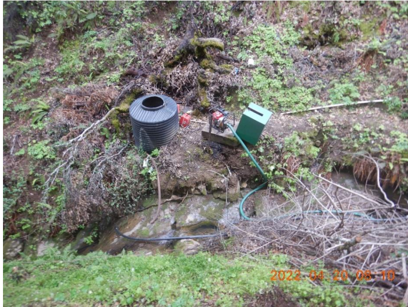
Photo 1— Looking south toward WQ1. A water tank and gasoline powered pump are installed on the right bank of a watercourse with flowing water. Pipes extending from the pump inlet extend into the watercourse.
