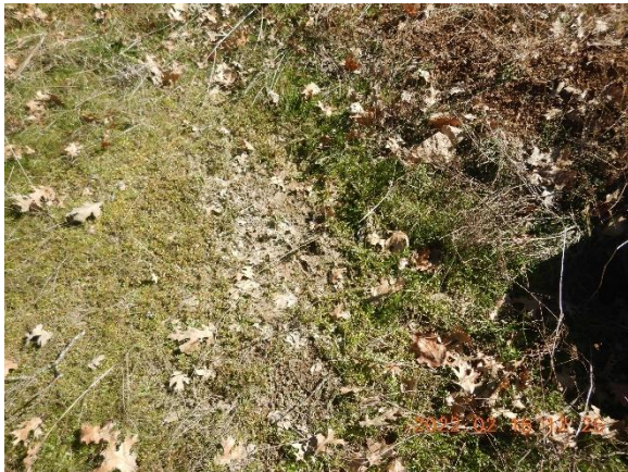
Figure 8. Culvert 2 inlet with signs of ponding.
