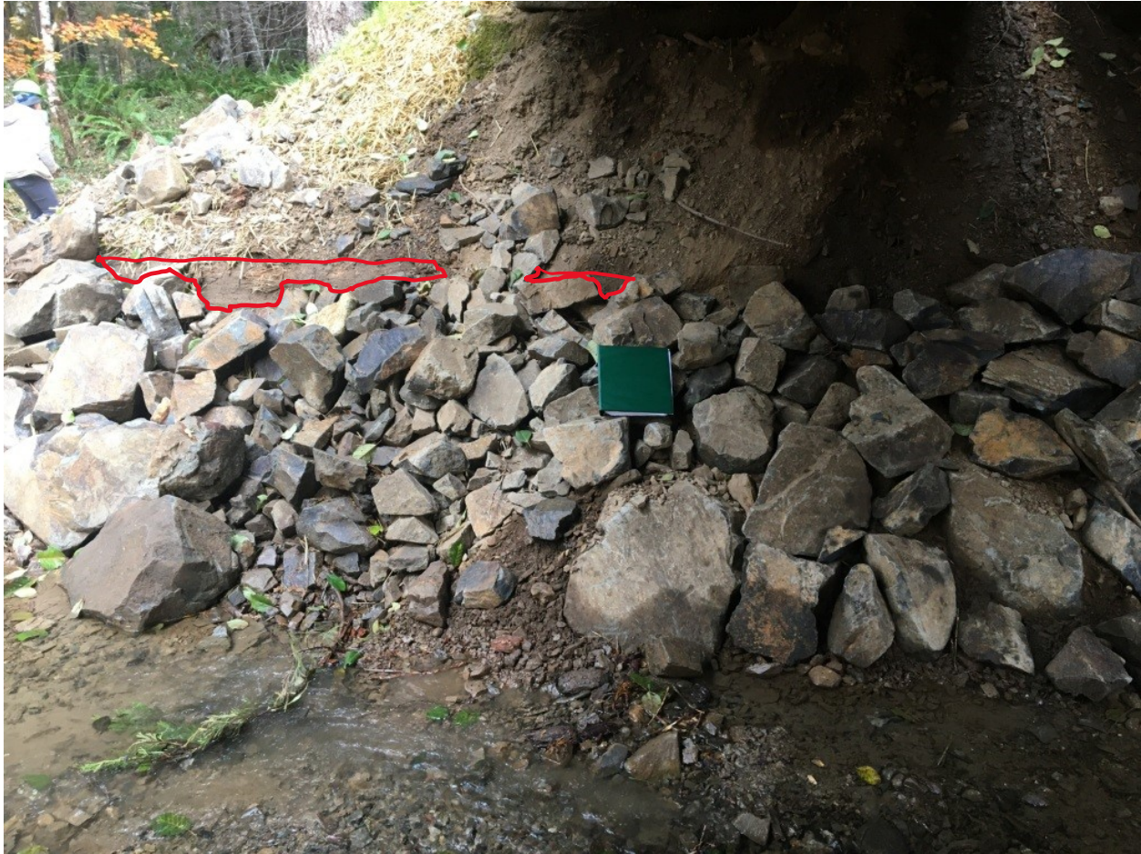
Figure 2: Abutment on the north side of RP1. Photo taken during the CDFW inspection conducted on November 10, 2020. Note log buried in the fill, outlined in red.
