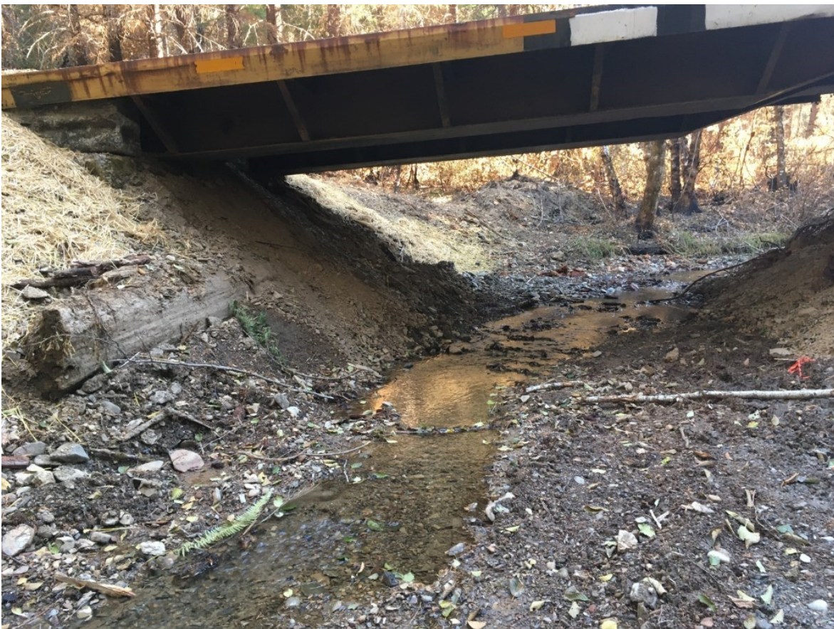
Figure 1: Looking upstream at the abutment on the north side of RP 1. Photo taken during the Regional Water Board staff inspection conducted on October 28, 2020.
