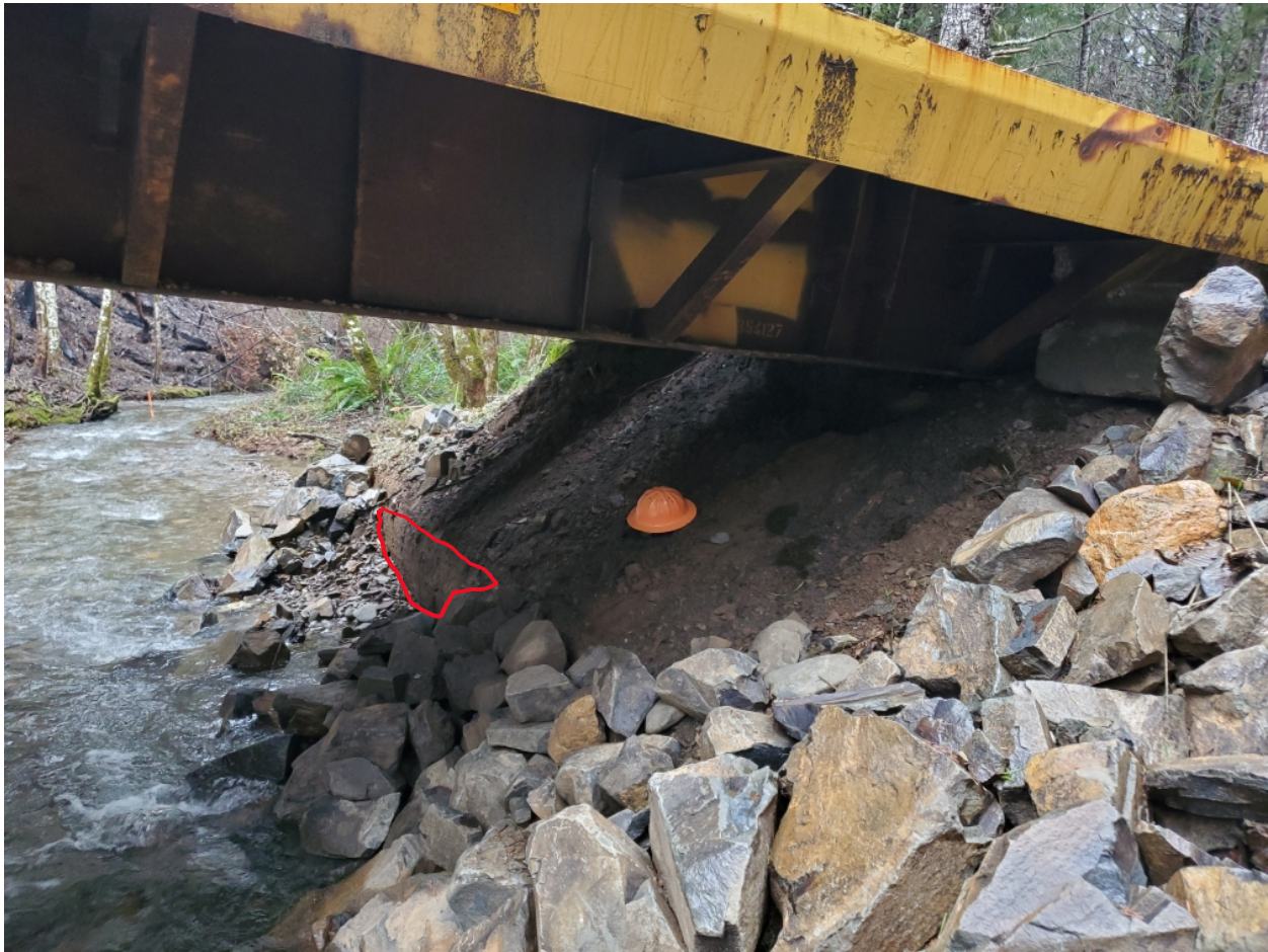
Figure 3: Abutment on the north side of RP1, showing erosion after storm damage (note exposed log outlined in red, also outlined prior to erosion on Figure 2). Photo taken by GDRC on January 21, 2021.
