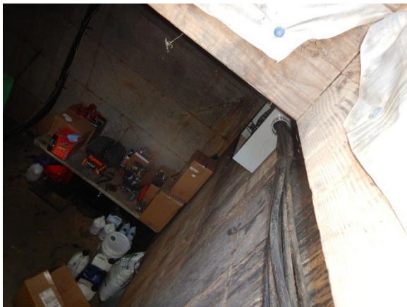
Figure 25. Via into buried container.
