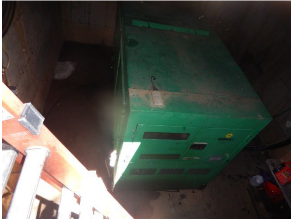
Figure 24. View of generator.
