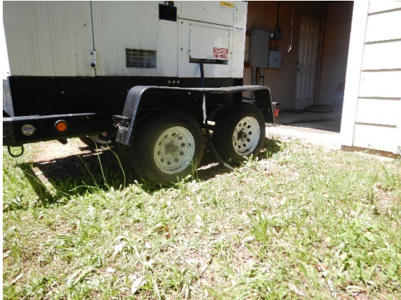
Figure 6. Generator on trailer by shed.
