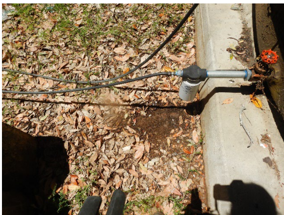
Figure 8. Fuel filter on fuel storage tank with stain on dirt at filter.
