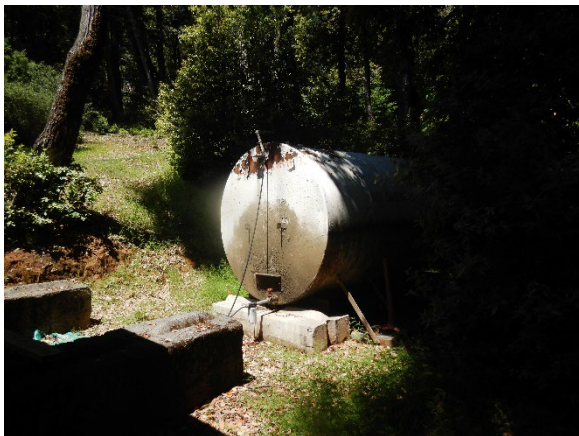
Figure 7. Fuel tank behind shed.
