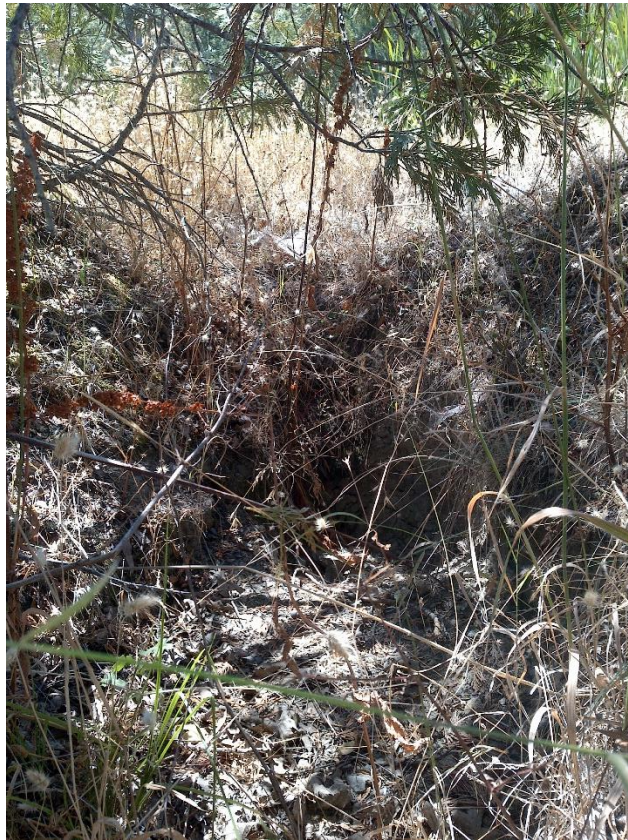
Photo 7— Hole scoured into the reservoir berm at WQ4.
