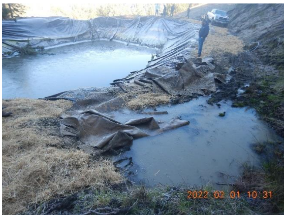
Figure 11. View of pond seep along cut bank.
