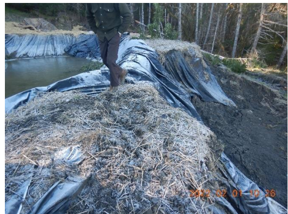
Figure 7. View of remaining berm between failure of Pond 2 interior.
