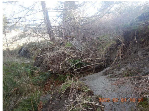
Figure 19. Saturated soil release from area of recent vertical displacement.
