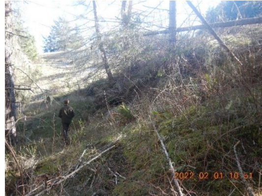
Figure 18. Slope at toe, eastern side of recent berm movement, and jack-strawed trees.
