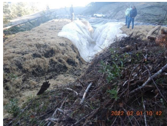
Figure 13. The pond outlet, recently deepened in an emergency effort to lower the overflow.
