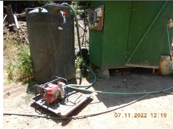
Photo 1: water storage tank and pump at inspection point WQ1
