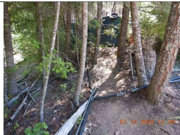
Photo 6: water storage tanks at inspection point WQ3
