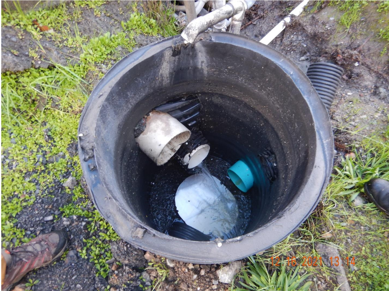
Photo 15 – Stormwater junction box east of stainless steel tanks adjacent to Pond 1.
