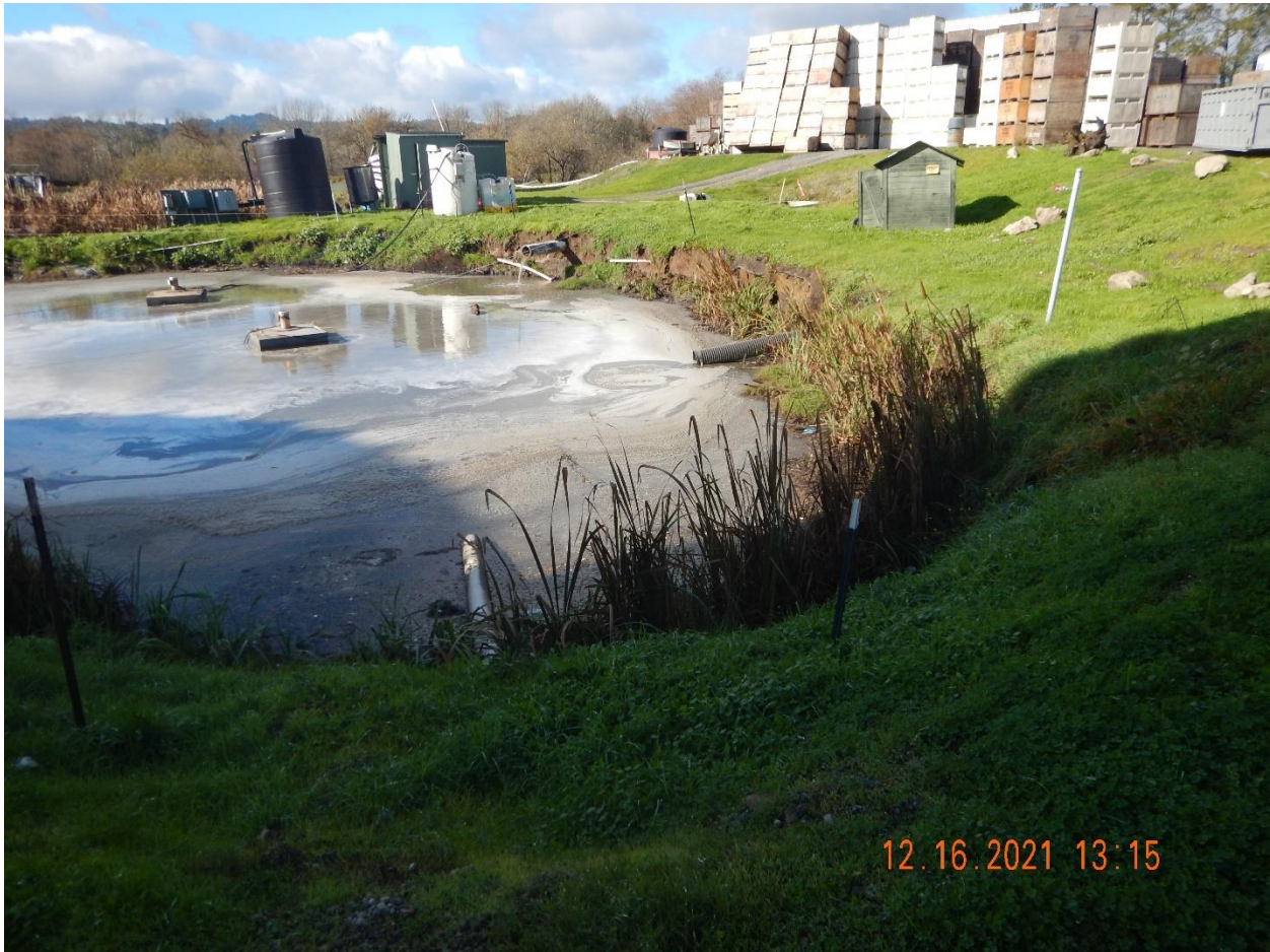
Photo 16 – Discharge pipes to Pond 1. Photo taken from southeast corner of Pond 1.
