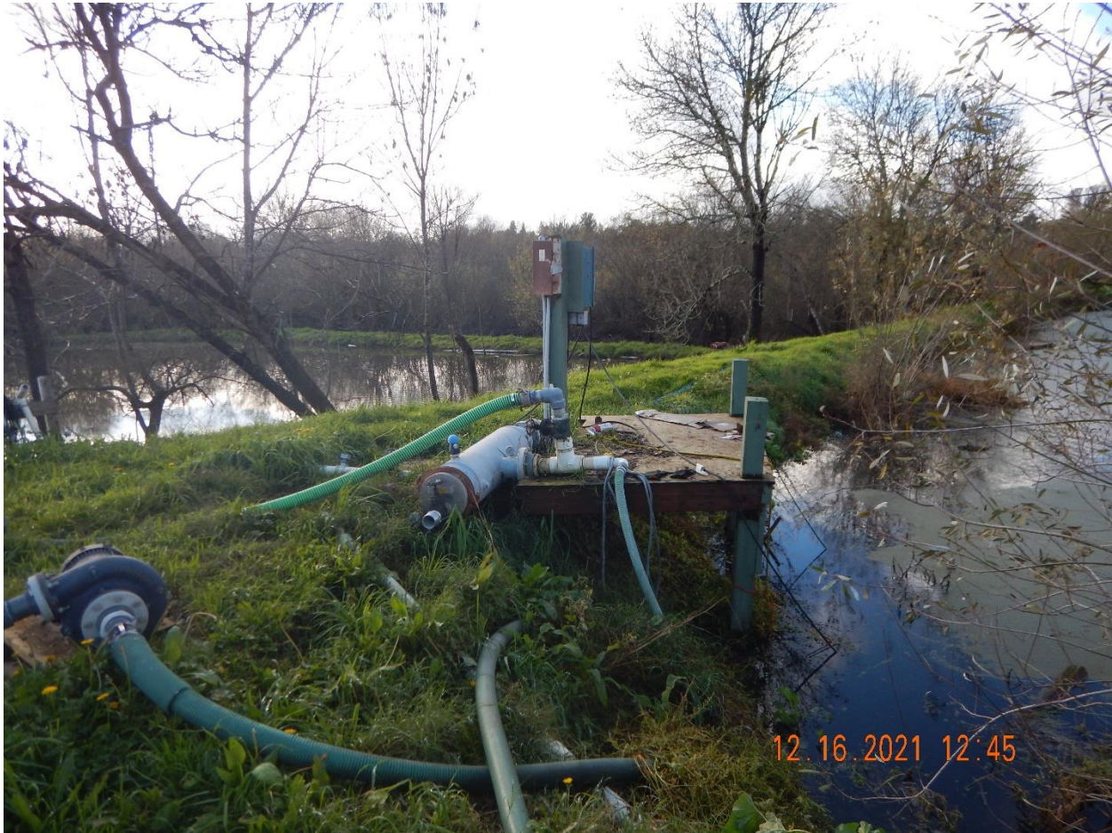
Photo 10- Southeast corner of Pond 3, wooden platform with electric panel and pump. Flooded south irrigation field in background. Flow meter area. Photo taken facing southwest.
