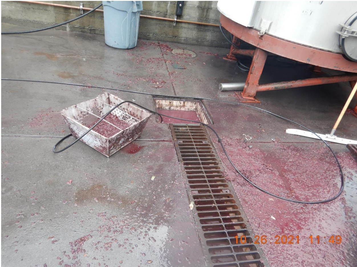
Picture 4- View of the wastewater trench drain near the crush pad area. Red staining was observed on the ground and inside of the trench. Picture taken by Farzad Kasmaei.
