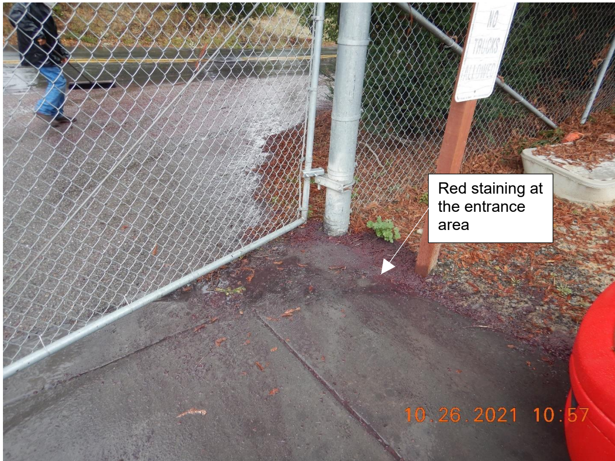
Picture 6- View of the red staining on the ground within the entrance area (Facility's gate) where the spill has flowed to the adjacent road. Picture taken by Farzad Kasmaei.
