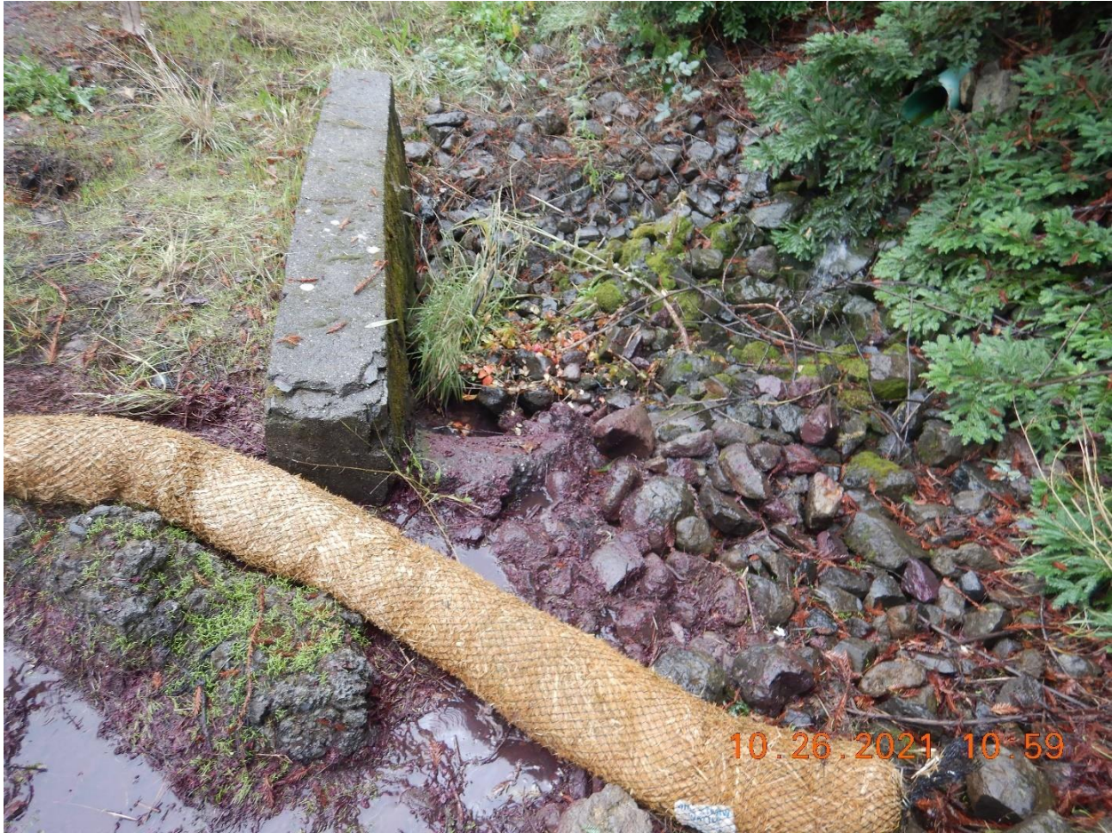
Picture 9 - View of red staining in soil within the roadside trench area and installed wattle. Picture taken by Farzad Kasmaei.
