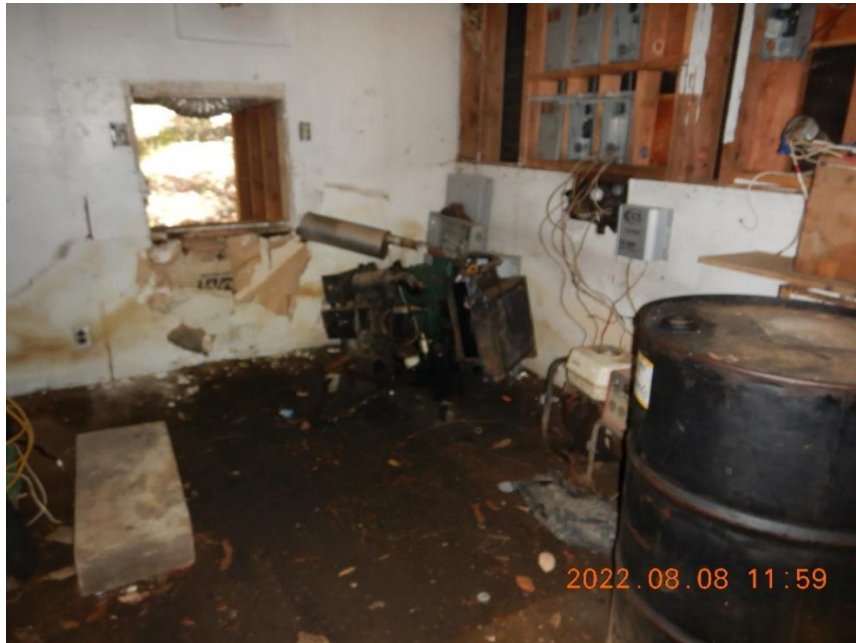
Photo 15—Looking inside generator shed located at WQ10. The wooden floor is stained with oil.
