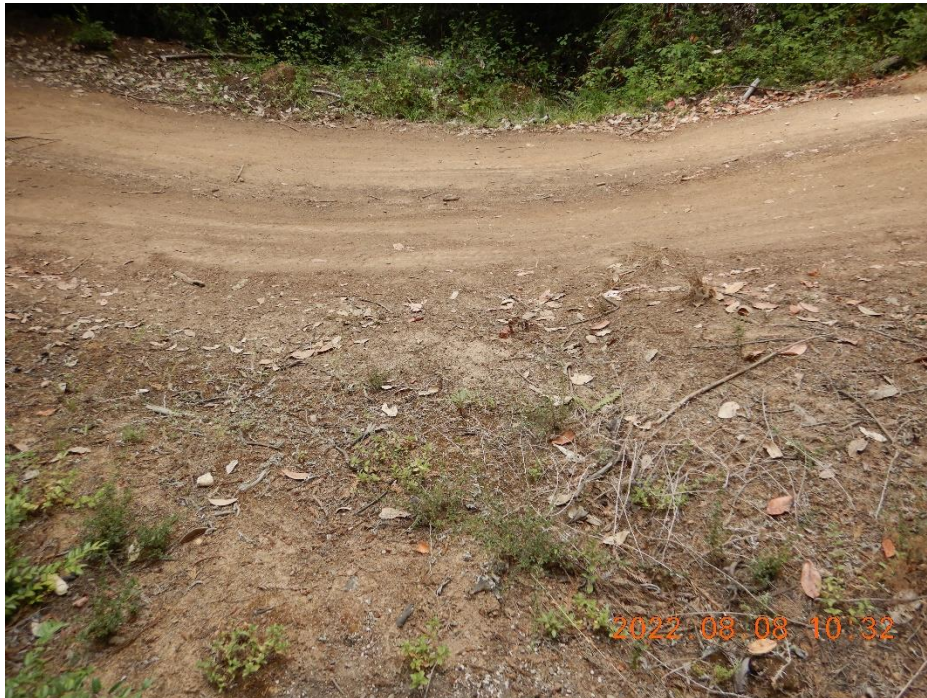
Photo 7—Looking south at a road fording a watercourse at WQ3. A channel scoured from concentrated stormwater is visible in the foreground of the image and the topographic form of a watercourse with a duff covered bed is visible below the road in the background of the image.
