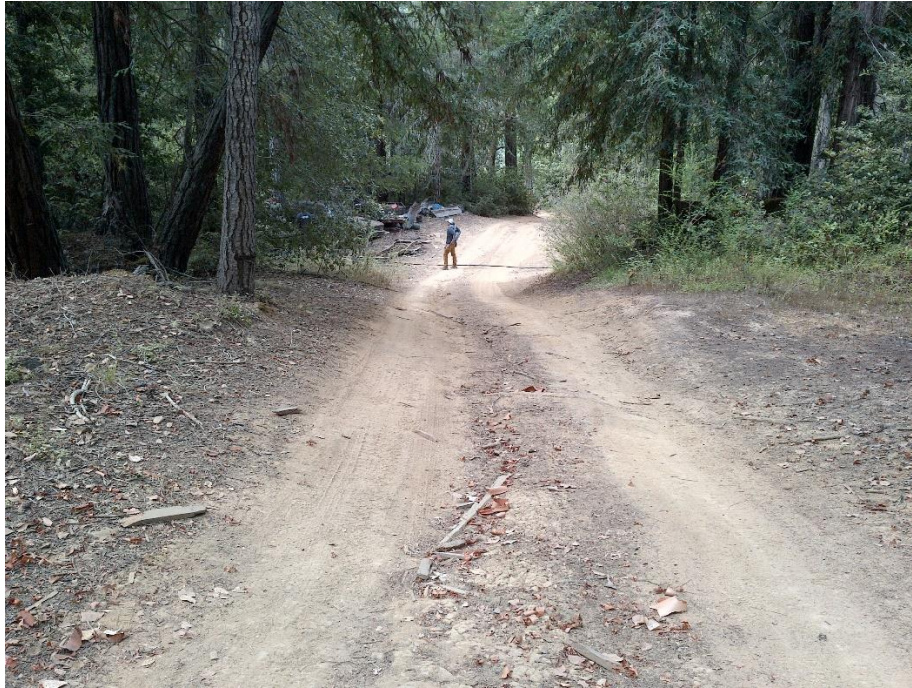
Photo 5— Looking south along road in the vicinity of WQ2. A scour mark is visible in the middle of the road where stormwater had concentrated and flowed downslope and past vehicles pictured in the top left of the image.
