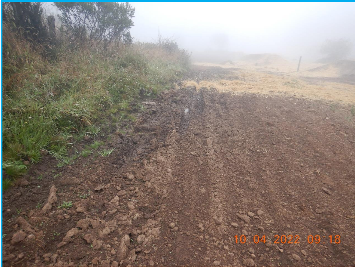
Photograph 2. Recently tilled dirt track. Note seep, ponded water, small sedges and rushes along track's edge. Note also graded jumps in background. Photographed by Amanda Piscitelli.
