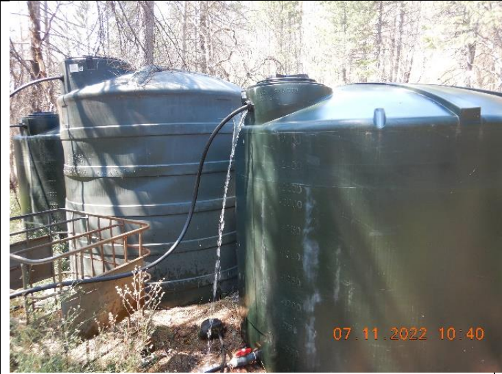
Photo 1: water storage tank at inspection point WQ1
