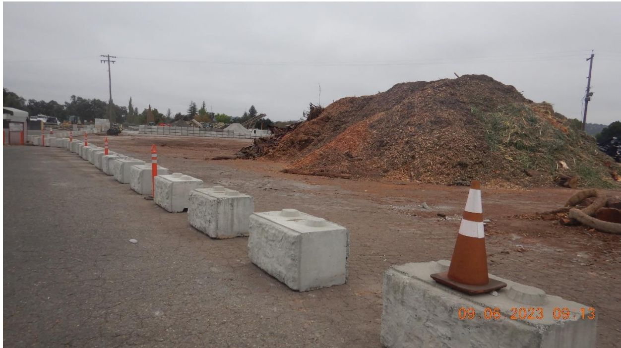
Picture 6 – Looking northeast at the wood chips storage area where large wood chips stockpiles are stored adjacent to the western property line with no effective and adequate perimeter control BMPs. Picture taken by Farzad Kasmaei.
