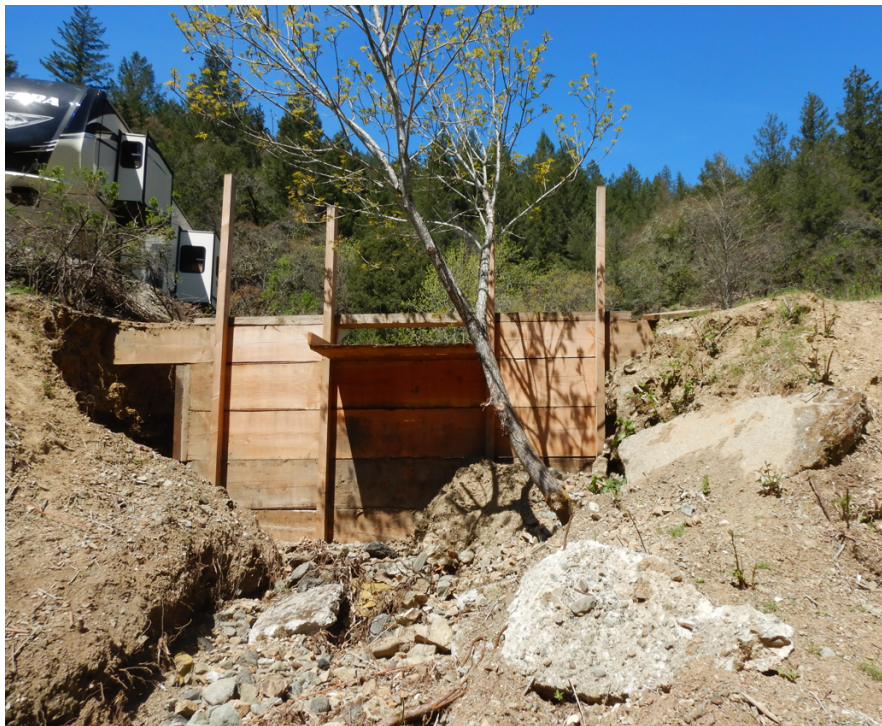
Photograph 2: Photograph taken by Mr. Greer. The photographer is looking up the tributary showing the failed wooden dam. Bank failure can be seen on the left side of the dam where the bank eroded away.
