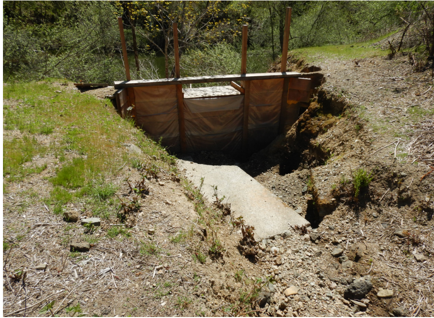
Photograph 1: Photographer is looking down the unnamed tributary to Outlet Creek showing the failed wooden dam. Large slabs of concrete are buried in the elevated flood terrace.
