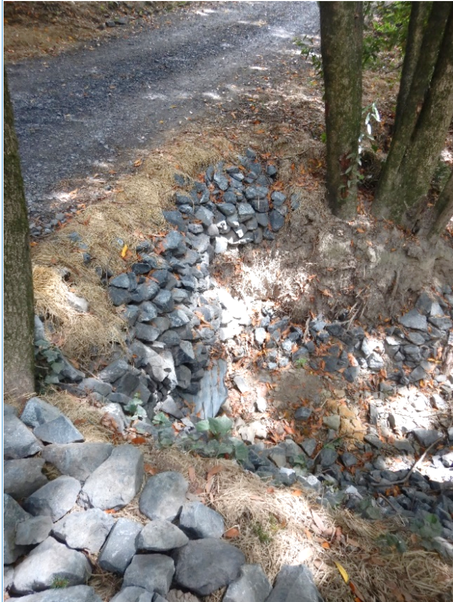
Photograph 5: Near-vertical road fill face lined with RSP. Note RSP in stream and pile of RSP in foreground at risk of discharging into stream.
