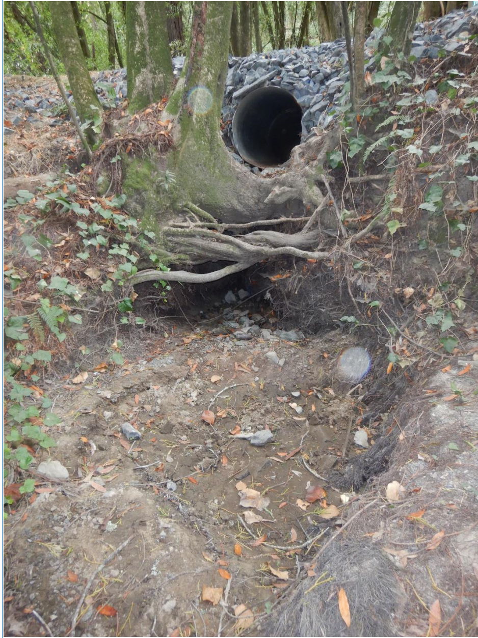
Photograph 4: Culvert outlet not at channel grade with steep road fill face armored with RSP. High flow is eroding the stream bed, forming a plunge pool, and exposing roots and tree trunks.
