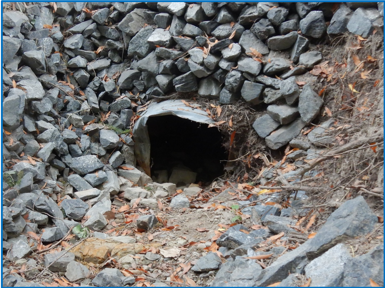
Photograph 3: Rock and debris obstructing partially crushed culvert inlet.
