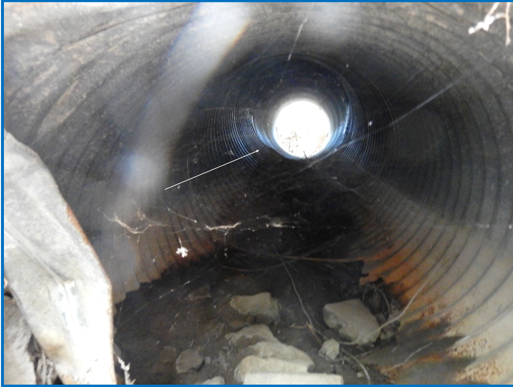
Photograph 6: Rust line approximately 10-12 inches wide extending from culvert inlet to outlet. Arrow identifies bend/kink in culvert creating reverse flow.
