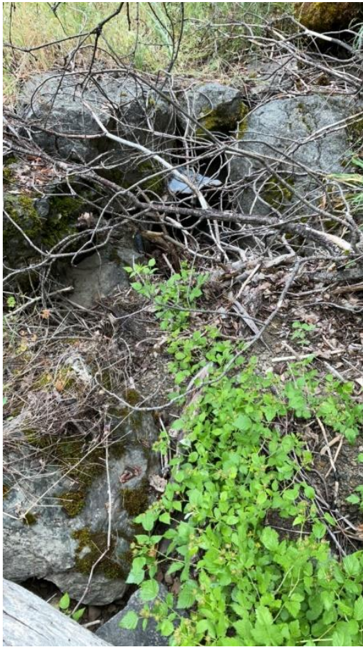
Figure 33. Inlet x3, undersized culvert
