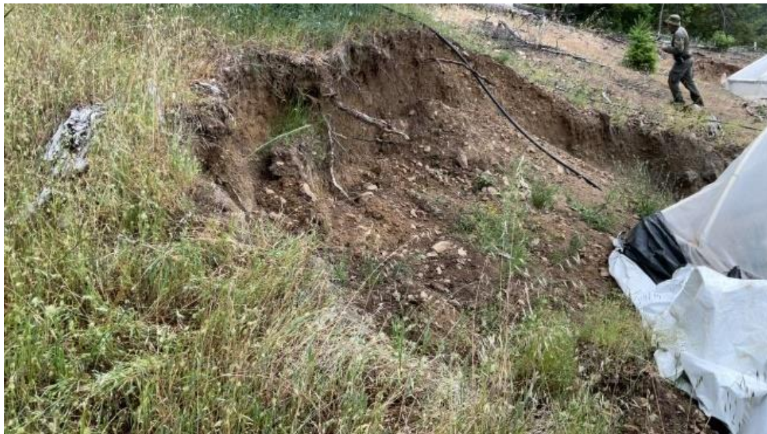
Figure 38. Cut bank failure associated with CA3.
