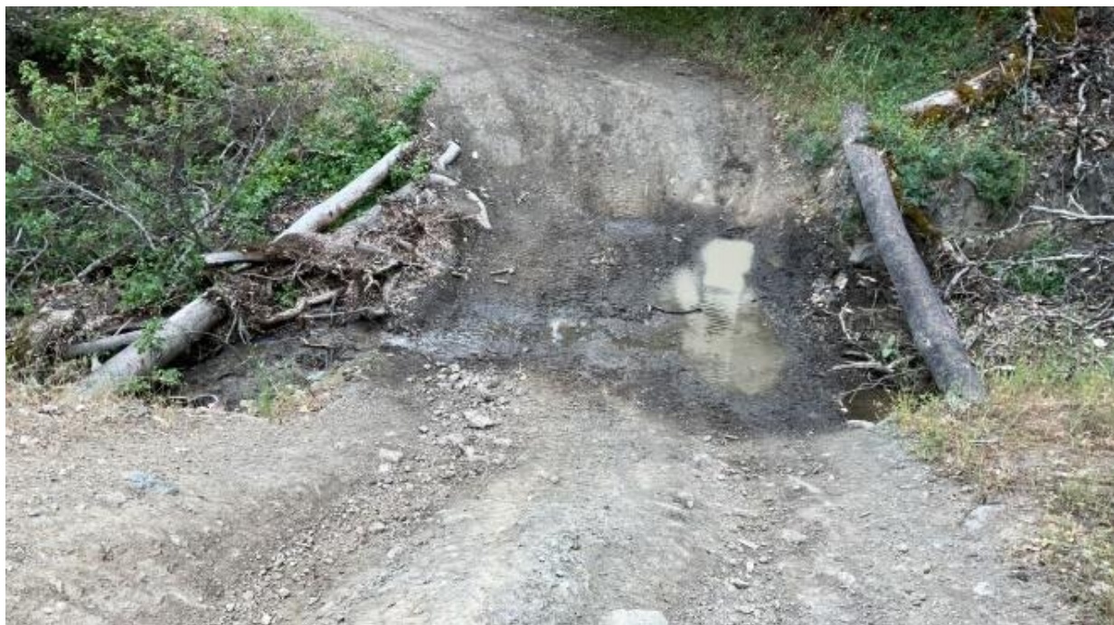
Figure 53. X7. Ford over a blue line Class II watercourse with debris in channel and rutted mud tracks. Presence and use of the crossing result in sediment discharge. View facing SE, from left bank, downstream to left of photo.
