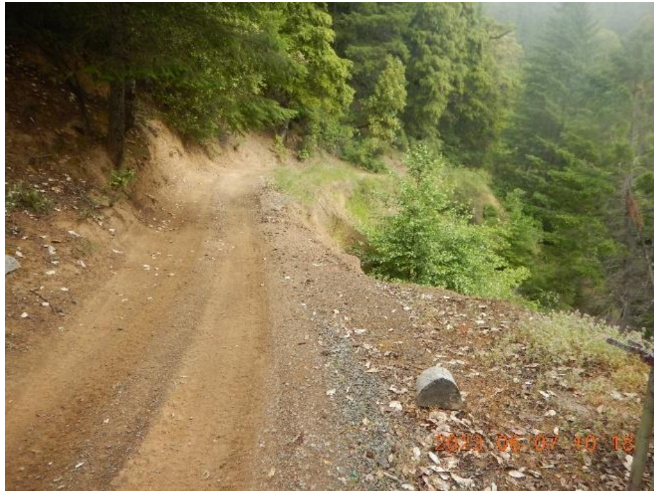
Figure 20. Slide associated with the failed slopes of the access road. Approximately 400 feet of road on the right bank of the watercourse is impacted by unstable slopes leading directly to the blue line watercourse.
