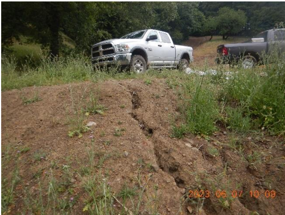
Figure 10. Eroded fill slope below X1, with delivery to the class III watercourse.
