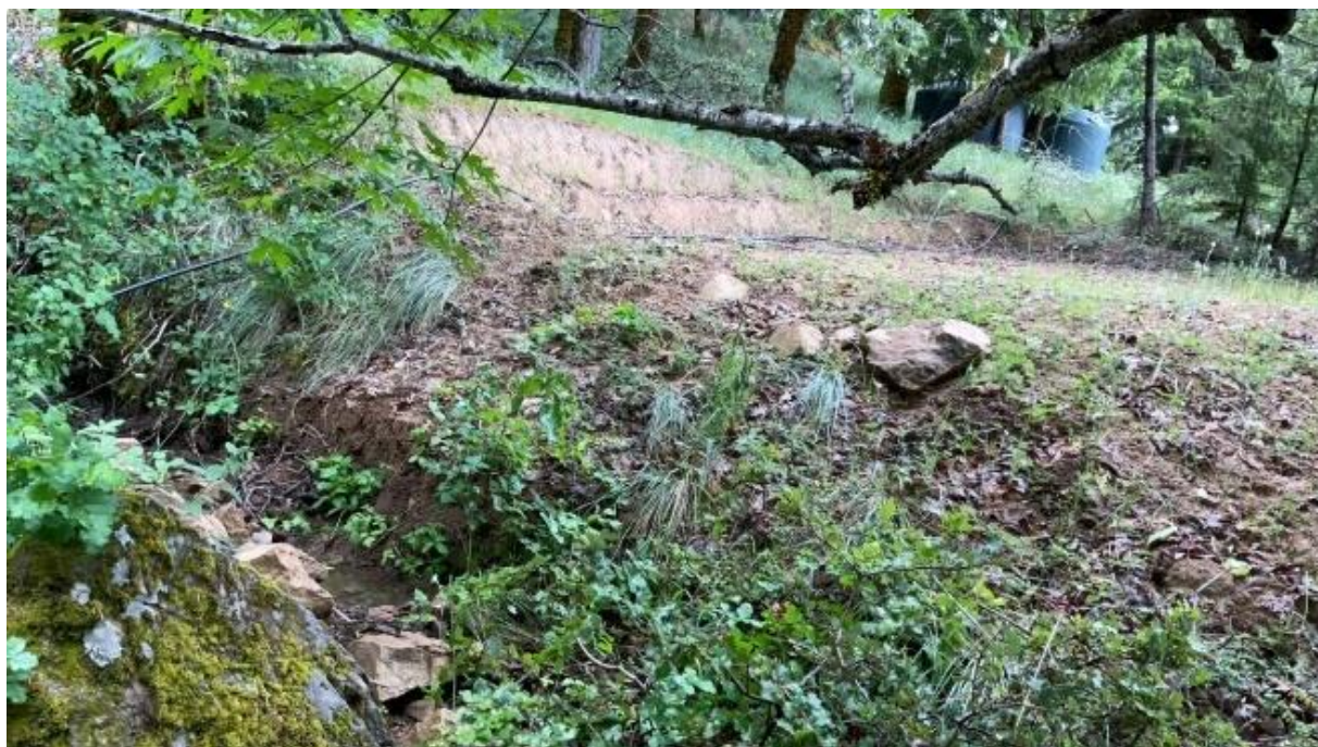
Figure 40. Graded area next to Class II watercourse has disturbed the stream bank and resulted in sediment delivery to the watercourse.
