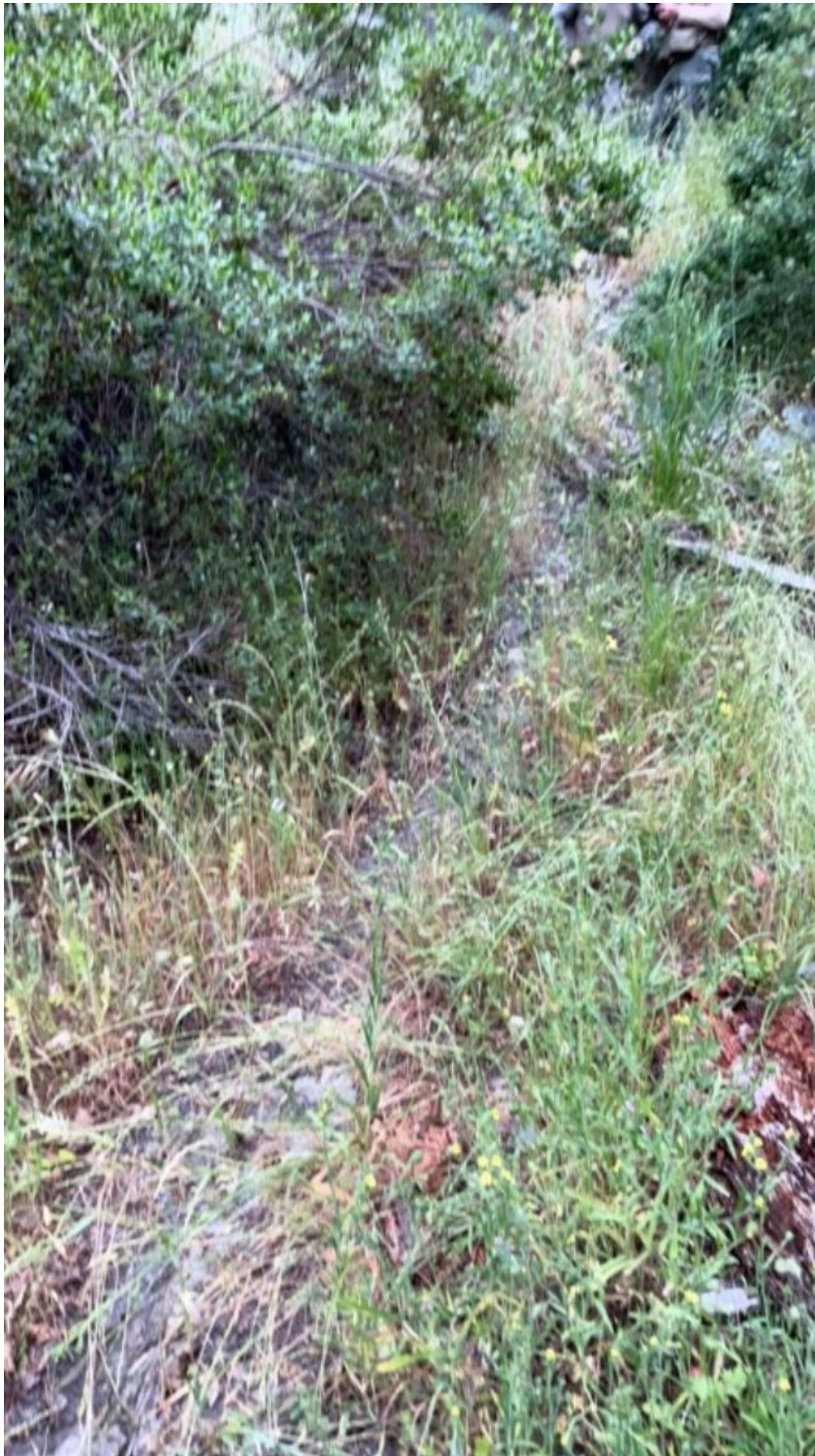
Figure 44. Below CA3, a steep road segment is undrained and surface erosion has resulted in sediment transport and delivery to the blue line watercourse.
