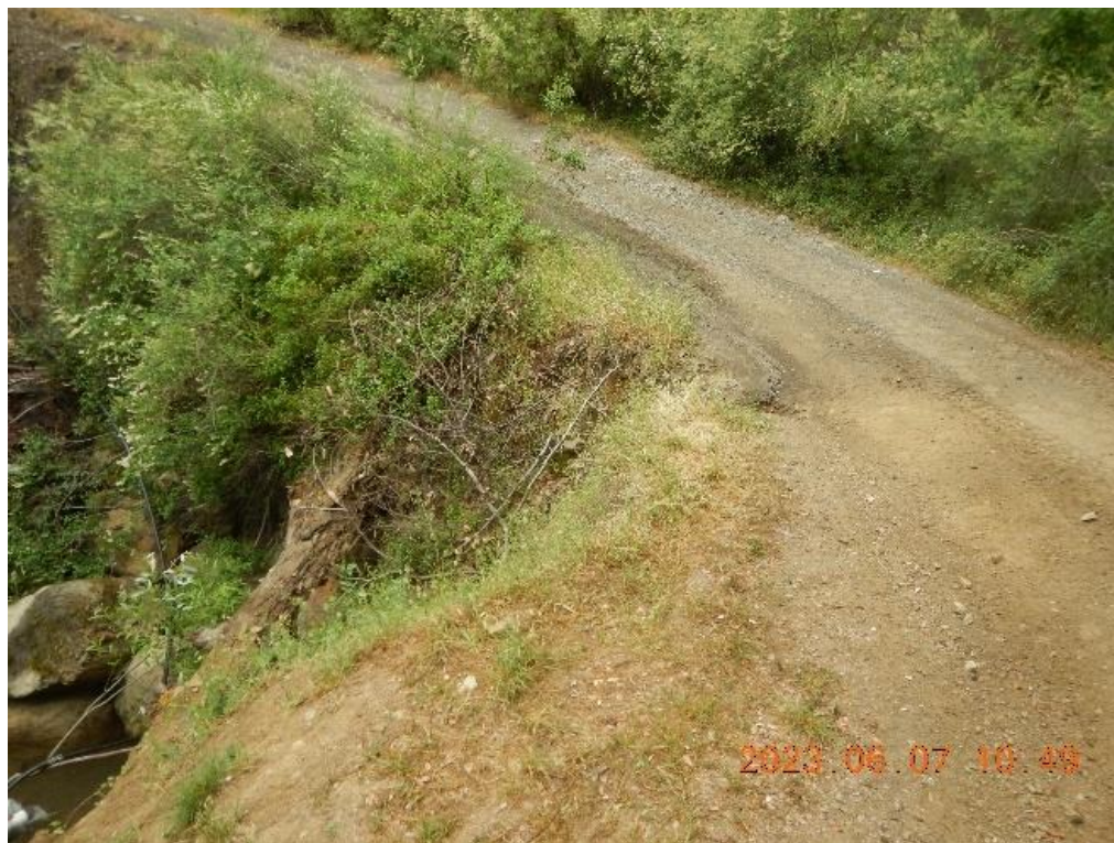
Figure 24. The road surface concentrates water and discharges stormwater to the watercourse at the outlet of X2.
