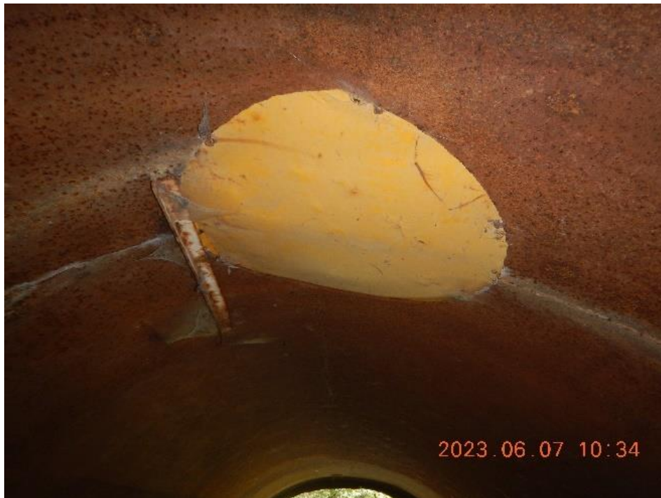
Figure 28. X2 culvert is fabricated from two metal cylinders with a seam in the middle and an opening that is patched with fiberglass.
