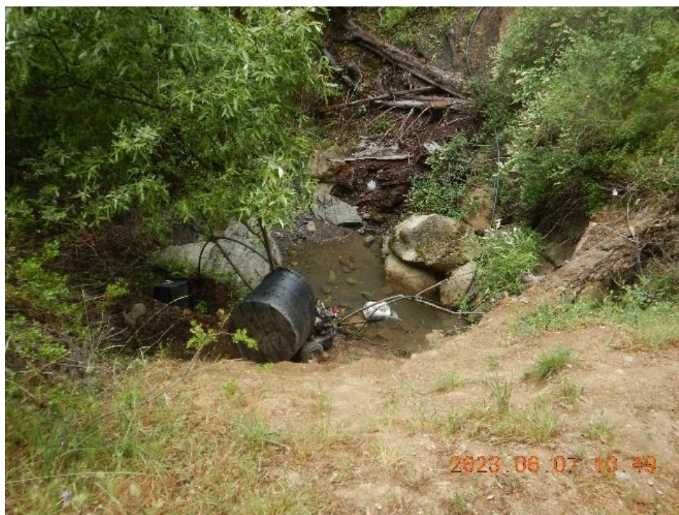
Figure 25. View downstream of X2 from road surface, with debris in stream.
