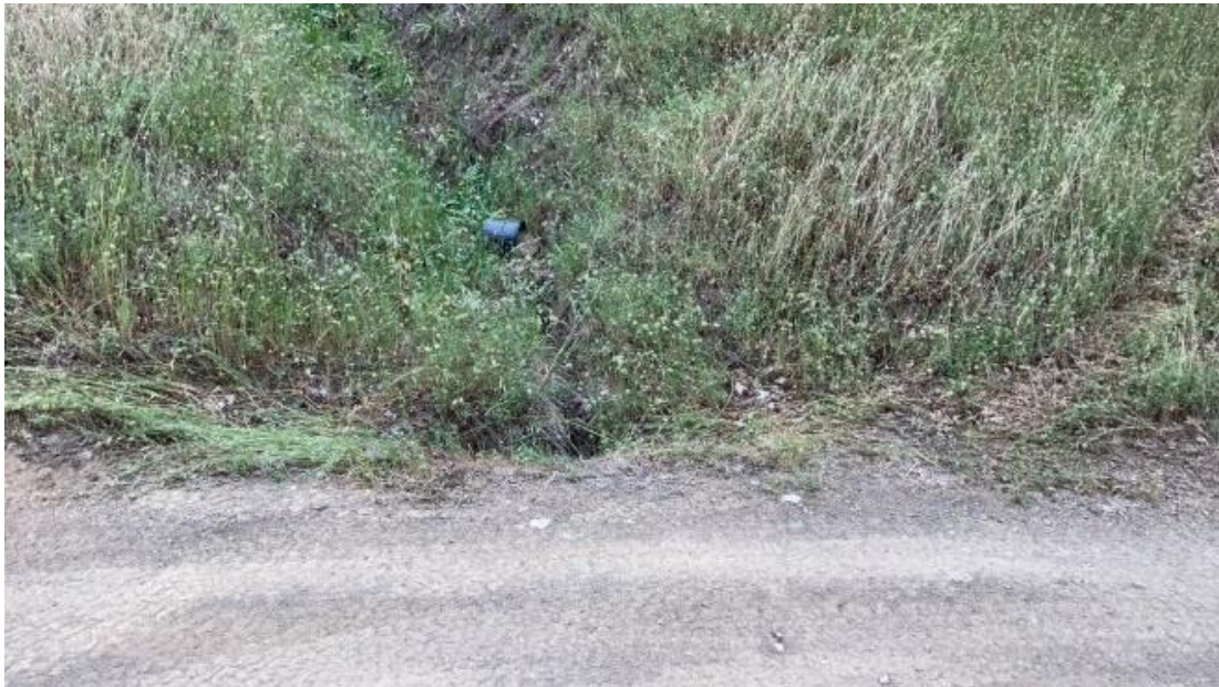
Figure 48. X4 inlet (facing SW). Undersized pipe, road sediment delivery.
