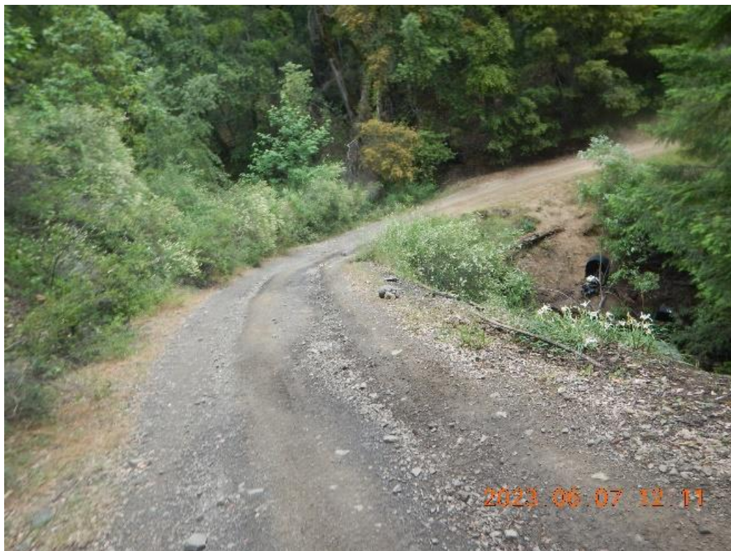
Figure 23. Outlet of X2 stream crossing and debris in stream.
