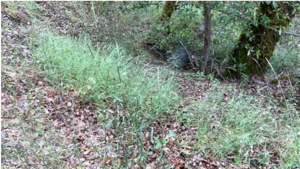
Figure 50. X6. 18 inch culvert perched 20 feet, undersized for channel, with road sediment delivery.
