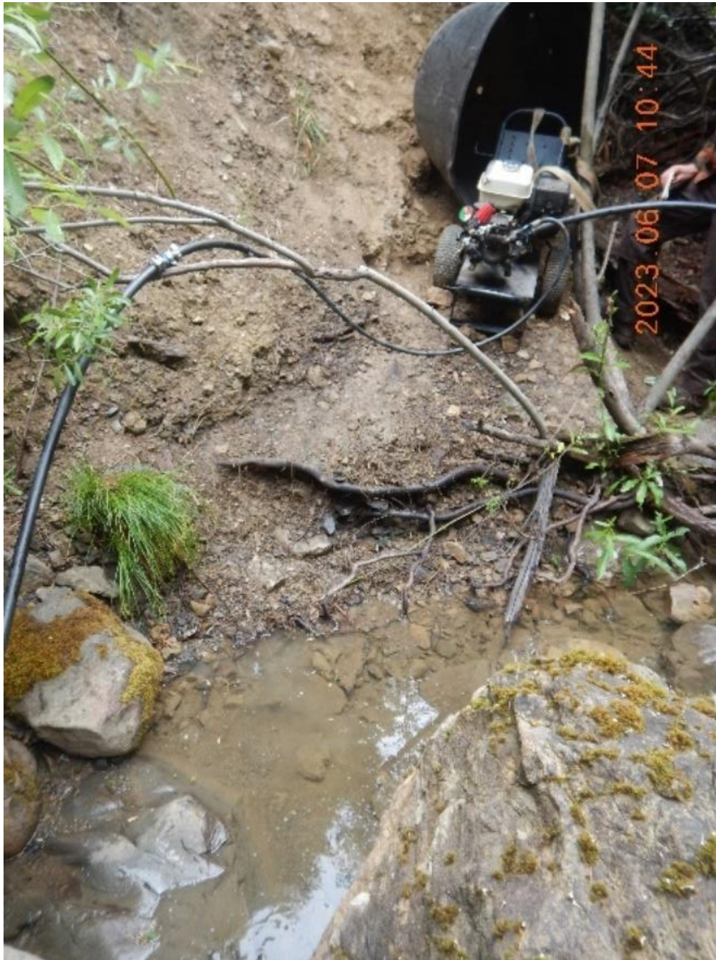
Figure 30. Pump at outlet of X2 culvert.
