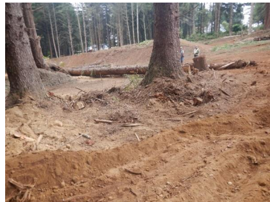
Figure 42. Loose soil in riparian area. Mound in rear of photo was recently constructed reportedly to build a largescale mound feature in the shape of a salamander.
