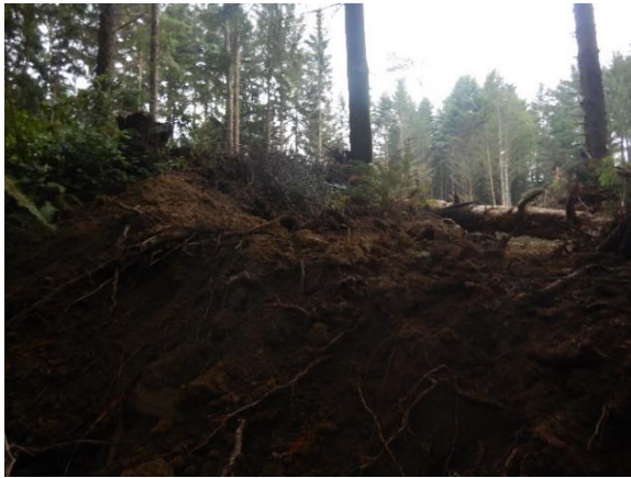
Figure 18. Fill next to watercourse and riparian area opened up by tree removal.
