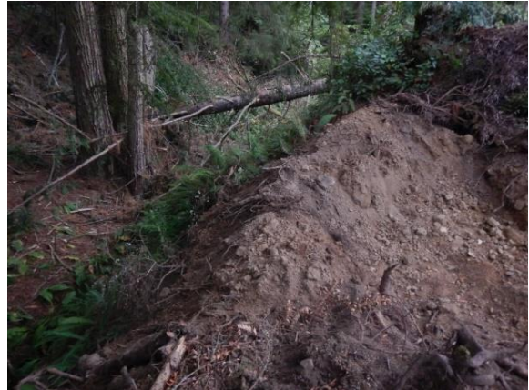
Figure 19. At WP956, the fill placed by the stream is approximately 25' L x 10' W x 12' high at watercourse side and 3' high on interior slope of fill.
