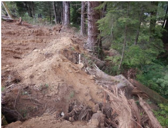
Figure 39. View of fill placed near WP956; material is loose and mixed with organic debris and is perched above watercourse.
