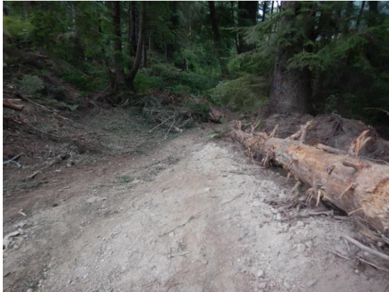
Figure 21. Road pushed through riparian area to watercourse at WP957.
