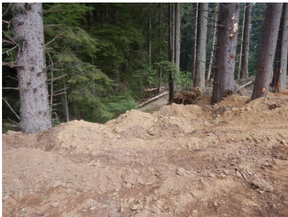
Figure 34. Fill pushed into riparian area.
