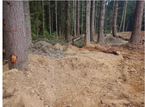
Figure 35. Fill pushed into riparian area.
