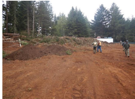
Figure 48. View of clearing and piling material, looking toward western Property boundary along Hunts Dr.
