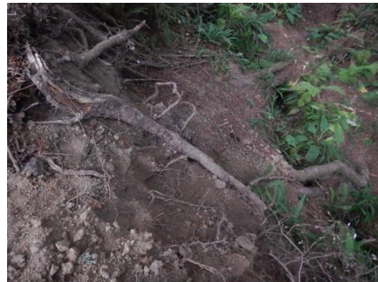
Figure 16. Sediment delivery path at WP956 to watercourse from perched fill.
