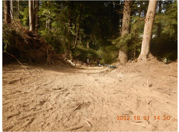
Figure 33. Road arrives at area A, where SHN and Ms. Rowland were preparing to begin sediment and erosion control work on the denuded stream bank.
