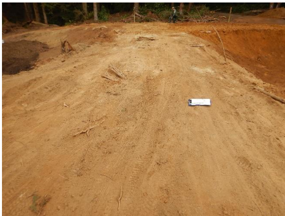
Figure 13. Looking downslope to watercourse in distance, pond berm on right (160' from stream bank), and lower mound "tail" on left (80' from stream bank). Buried slash is poking through the mound.
