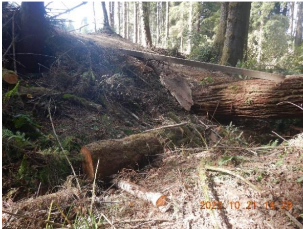
Figure 46. Fill has been pushed toward watercourse since my last inspection. This is the log spanner.
