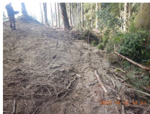
Figure 53. At area F, the fill pushed into the riparian area for 27', road goes back 46' to clearing. When asked about the construction, Mr. Gutierrez responded that he did it by hand.
