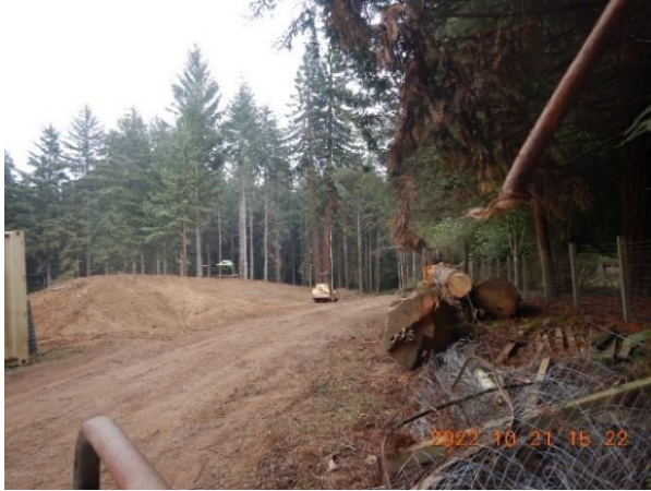
Figure 4. View from gate of upper mound and access road that parallels the southern parcel boundary to the watercourse. The mound was larger than I observed last inspection. Mr. Gutierrez claims that the slash is buried in the mound.
