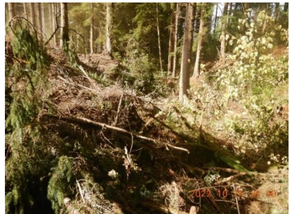
Figure 44. Looking downstream to area E, the channel is covered in slash.
