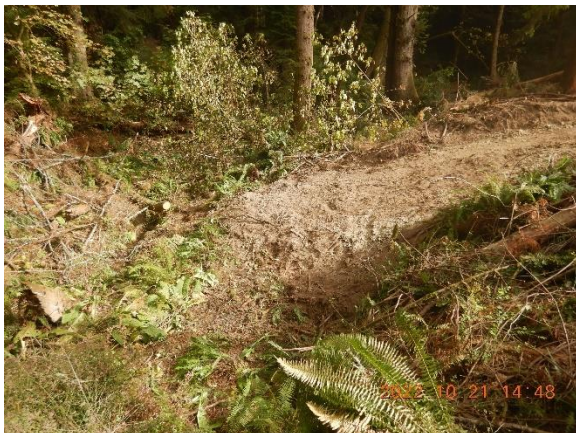
Figure 41. Area D. Channel is located where cut branch end is visible, left of center. Downstream is right to left. The new road fill is pushed from right, toward watercourse and onto a wet bench with skunk cabbage (obligate wetland plant).
