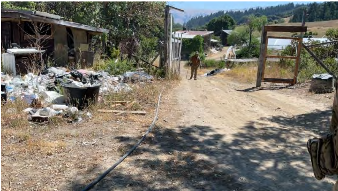
Figure 11. Point Feature 6 – the access driveway to the residence slopes down to the stream crossing and approximately three hundred feet of roadway is hydrologically connected to the stream crossing. The road is rilled and has deep dust. The road condition is threatened discharge of sediment to the stream at the crossing. At the top of the grade, plastic refuse is dumped and is not contained and could blow into the watercourse or other areas of the landscape.
