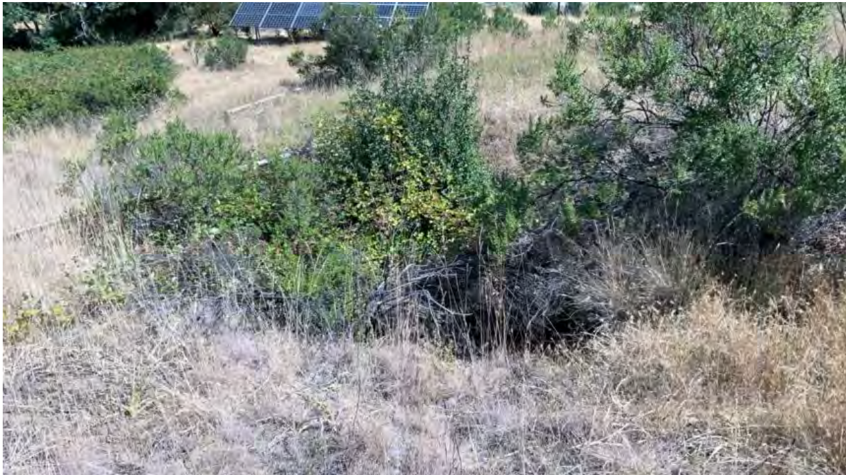
Figure 6. Point Feature 4 – erosional void associated with an older head-cut of the downstream channel.
