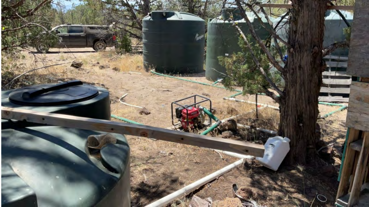
Figure 67. Water storage and feed tanks, and pump at location 3.
