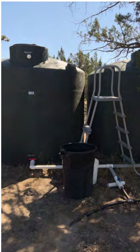
Figure 32. Water storage tanks at location 2.
