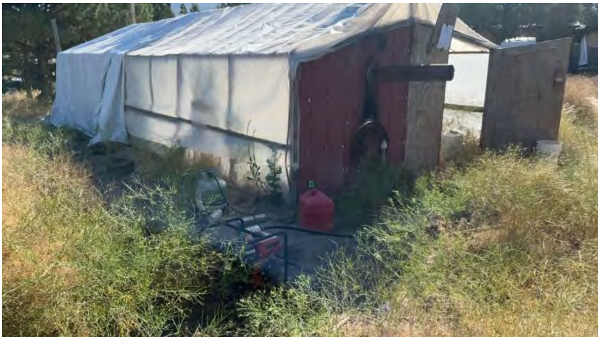
Figure 12. Gas pump leaking water near old greenhouse.
