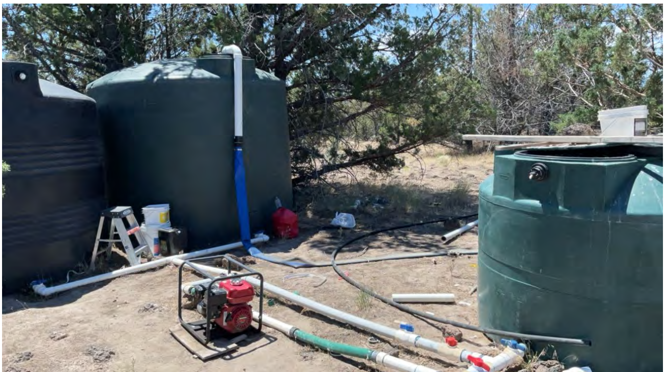
Figure 60. Location 6 water storage, feed tanks, fertilizer, and pump.
