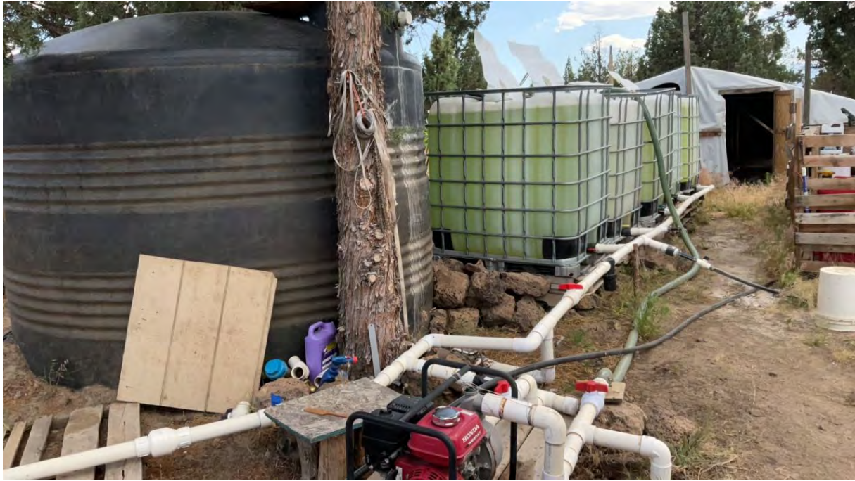
Figure 107. Water storage tank and feed tanks and pump at location 8.
