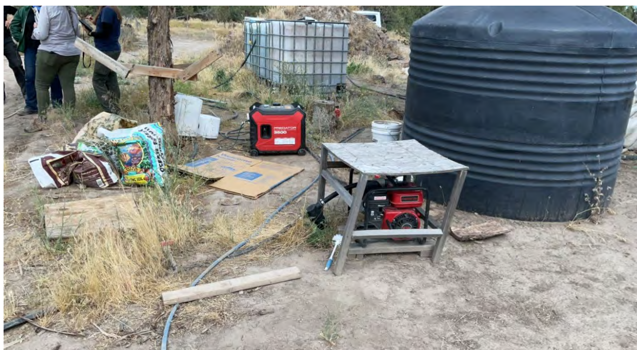
Figure 113. Feed tanks and pump at location 2.
