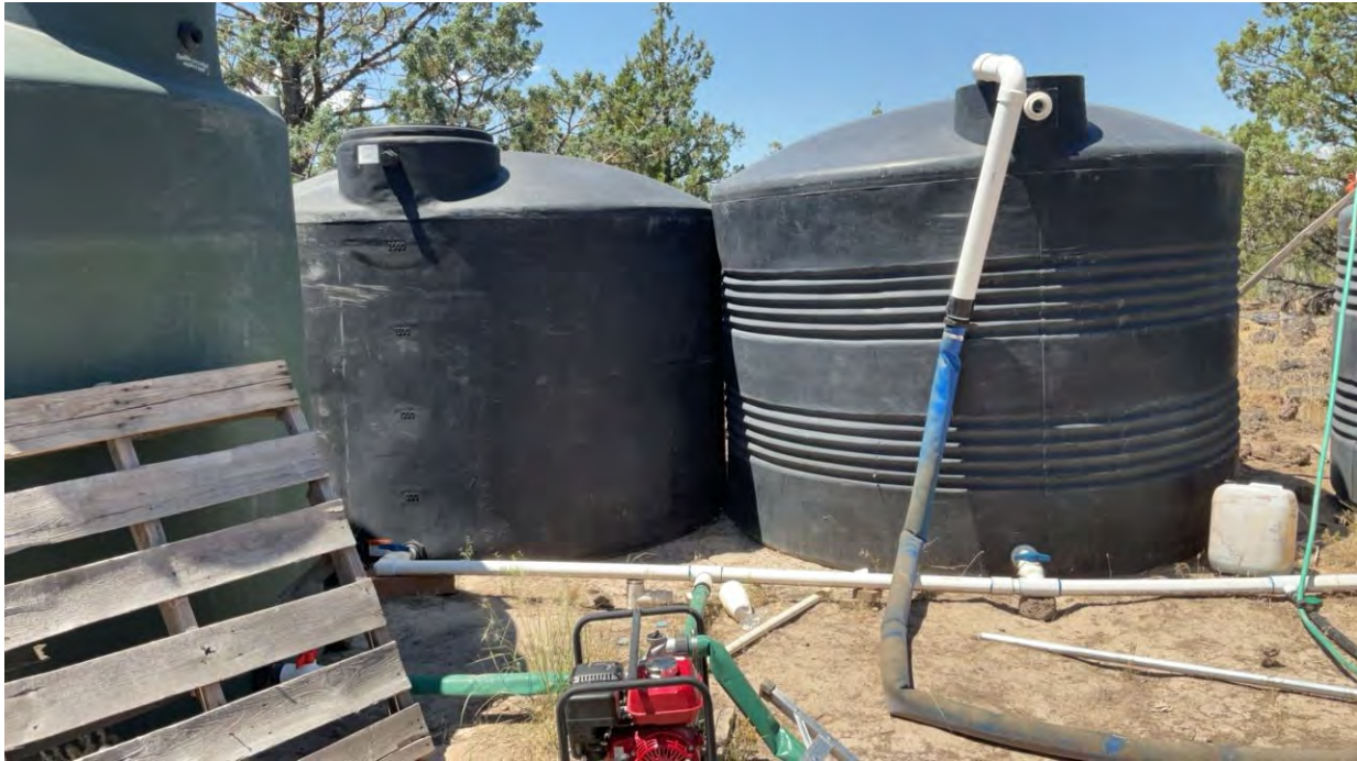
Figure 65. Water storage tanks and pump at location 2, similar to those observed at previous locations.
