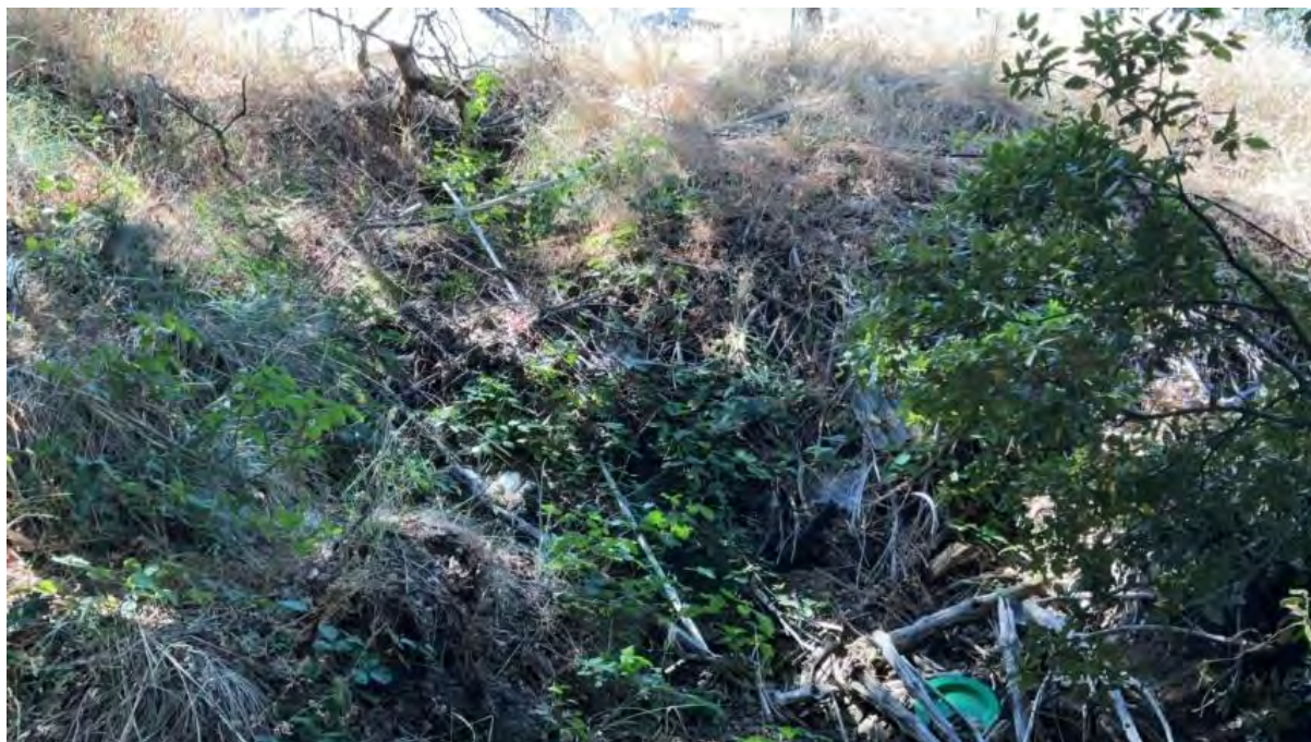
Figure 13. Line 6. Diverted watercourse delivers to a Class III watercourse in next drainage to east. There is a threat of additional sediment delivery along this new flow path.
