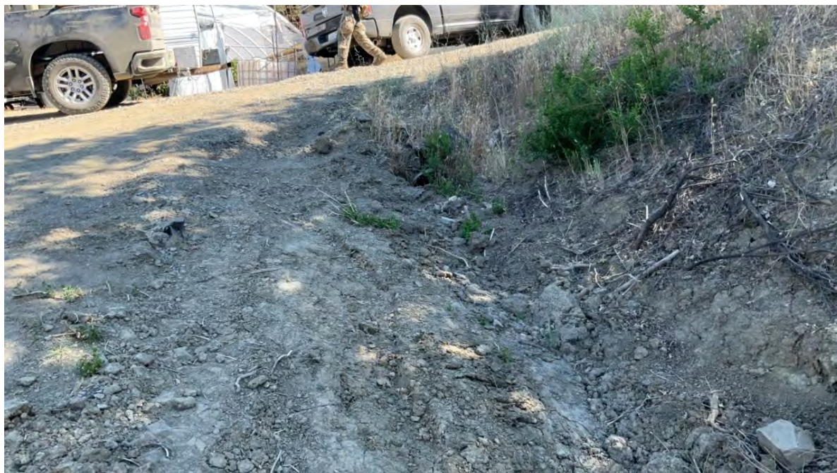
Figure 14. Line 8. Road-runoff delivers to a Class III watercourse.
