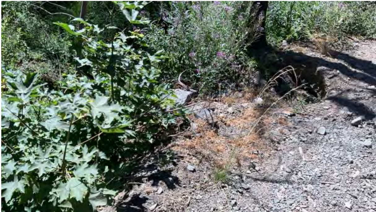
Figure 30. Point Feature 15 – Rubble on the left bank of the blue line watercourse with erosional void (actual discharge) and perched material (threatened discharge).
