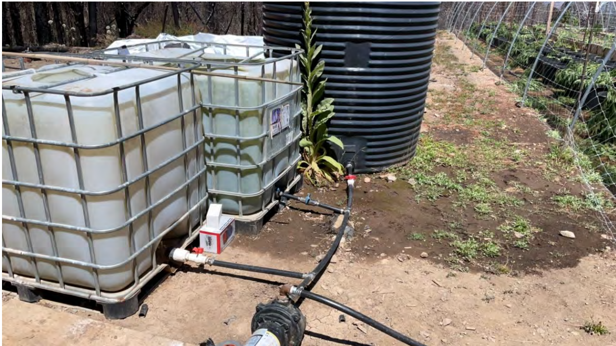
Figure 28. Polygon Feature 12 – water tank and feed tanks at cultivation area with signs of overflow.
