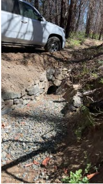
Figure 5. Point Feature 1- Recent rock work at inlet of culvert on side tributary along access road used to access cultivation area. The Regional Water Board has no record of application for authorization for instream work.
