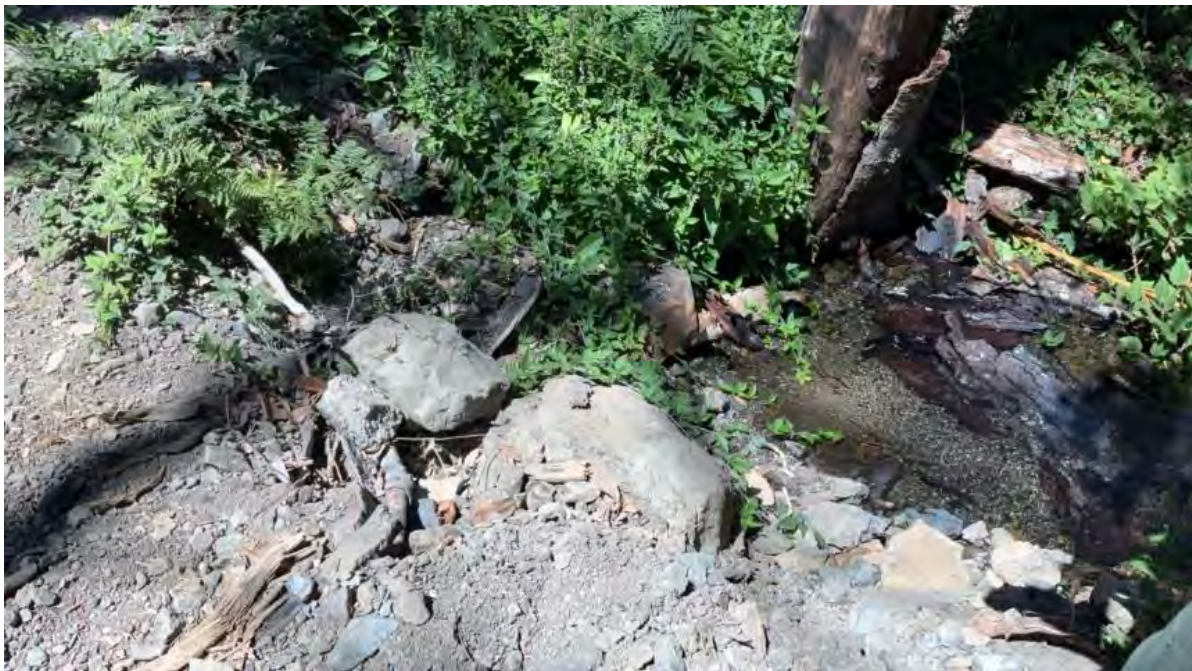
Figure 33. Point Feature 16 - CMP outlet. Threat of sediment delivery from road surface.
