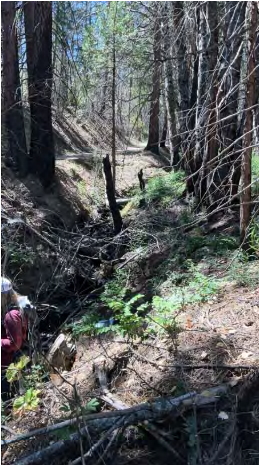
Figure 9. Point Feature 3 - Watercourse upstream of the point of diversion is impacted by sediment delivery associated with the road constructed within the riparian area of the watercourse.
