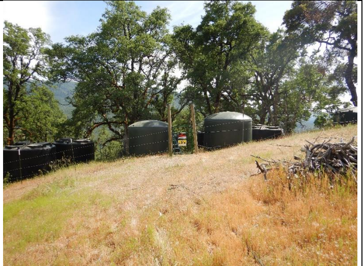
Photo 26: Water storage tanks at WQ17
