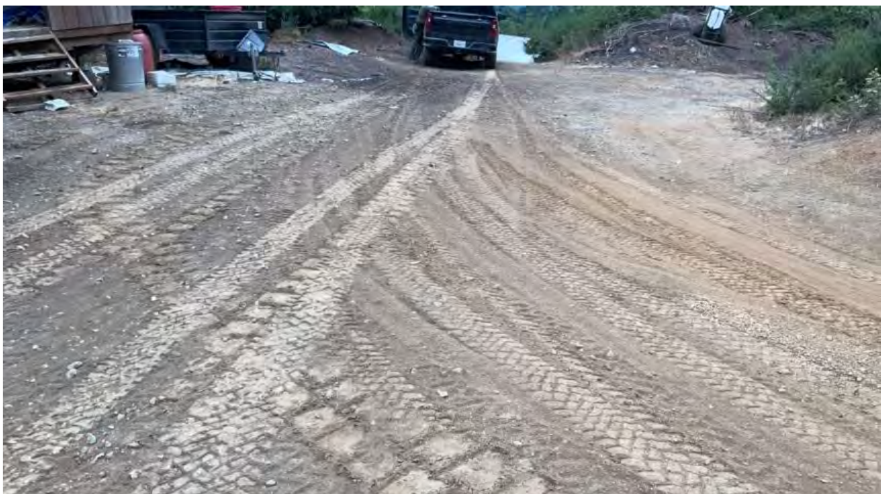
Figure 30. Point 14. Potting soil and spoils at top of steep road segment.
