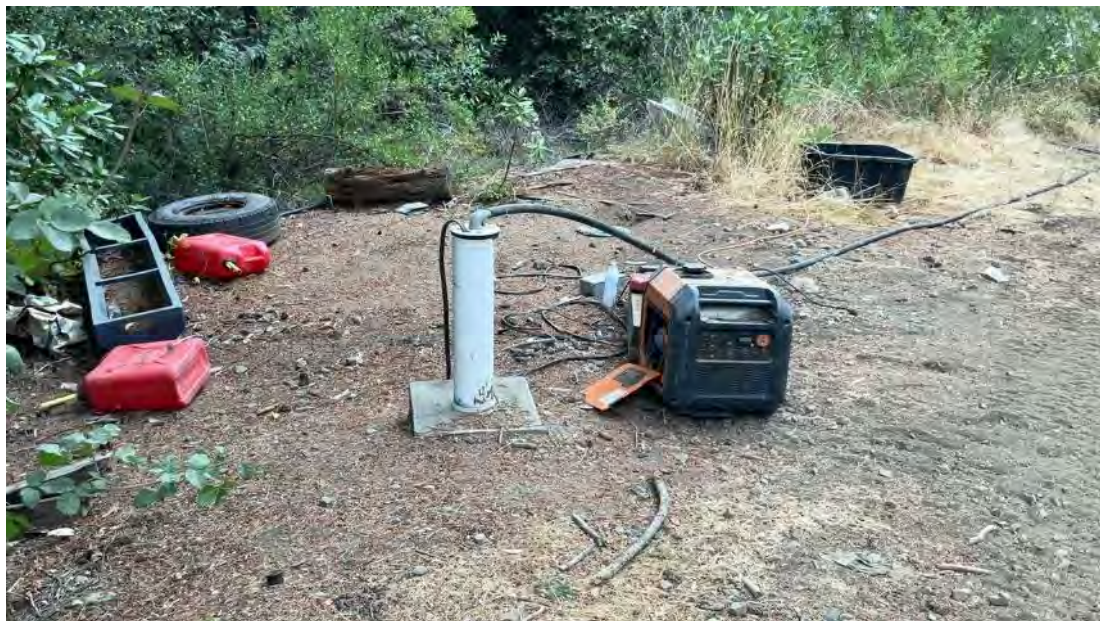
Figure 5. Point 1. Well with gas generator and gas cans.
