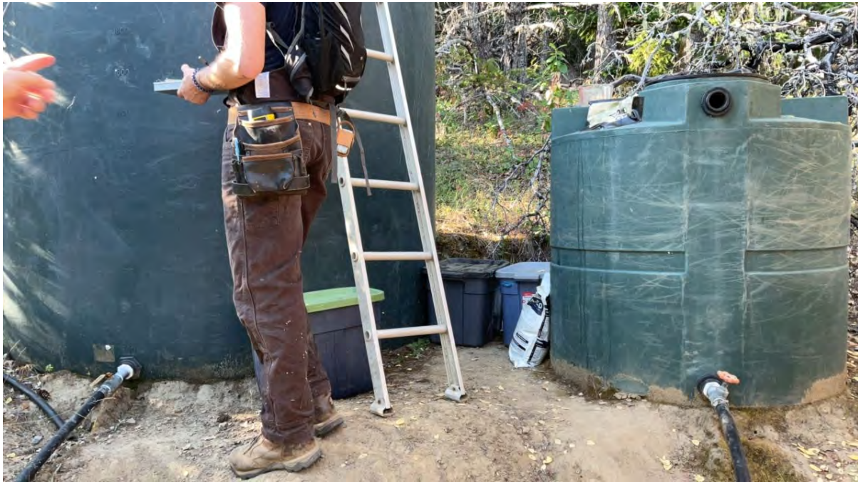
Figure 13. Water storage and feed tanks at Point 8.
