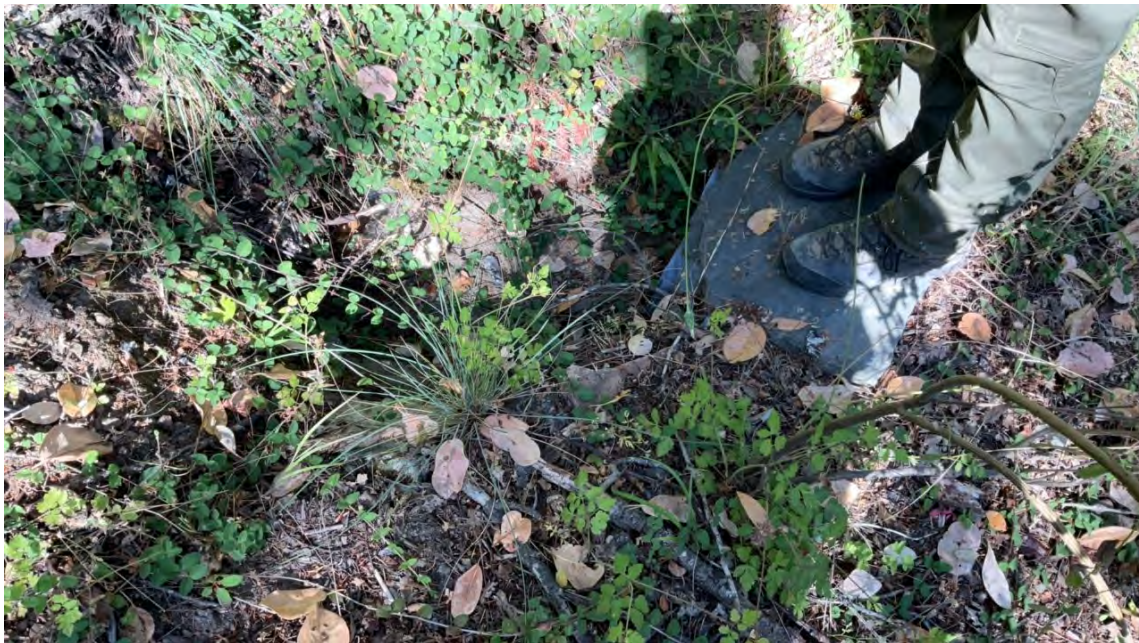
Figure 16. Point 10. Watercourse is intercepted by ditch; the ditch then enters the culvert, which delivers to a natural watercourse channel. The culvert is halfway filled with sediment. There has been road-related sediment discharge to the receiving watercourse and there is a threat of additional discharge.
