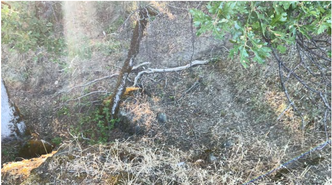
Figure 6. Polygon 1. Outlet pipe from pond discharges to a Class III watercourse.
