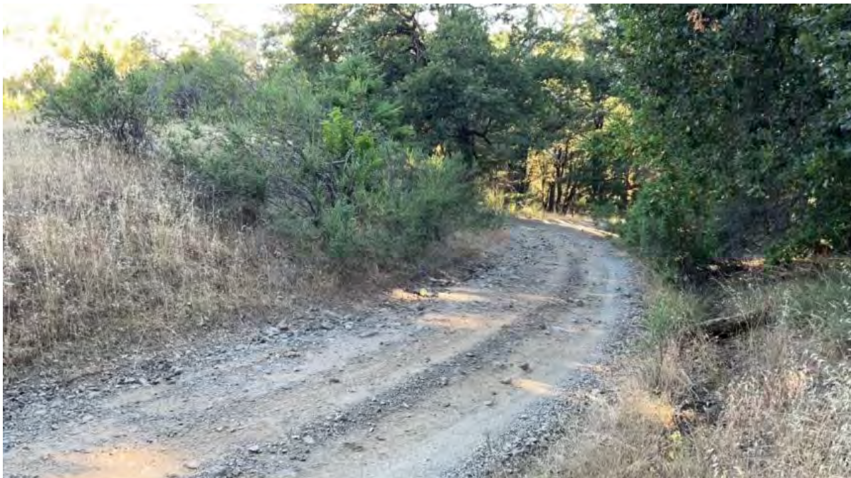
Figure 14. Line Feature 8. Road ditch and runoff with threatened discharge of sediment to watercourse.
