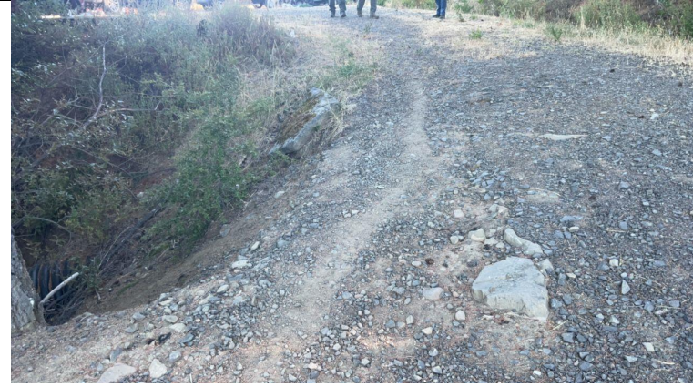
Photo Number: 4 Photo Description: Eroding dirt road prism. Facing West
