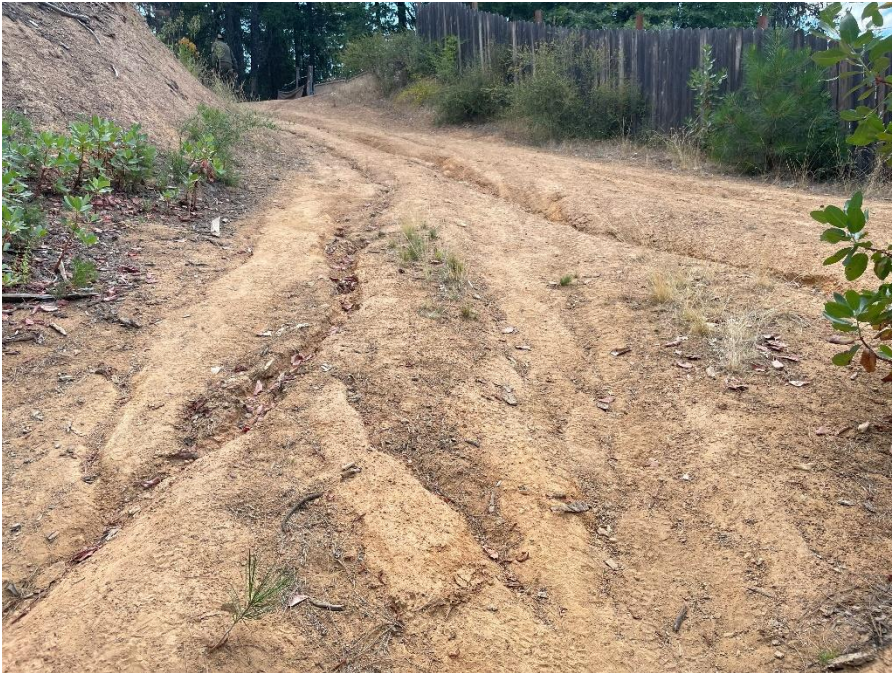
Photo 1: Dirt access road with rutting.
