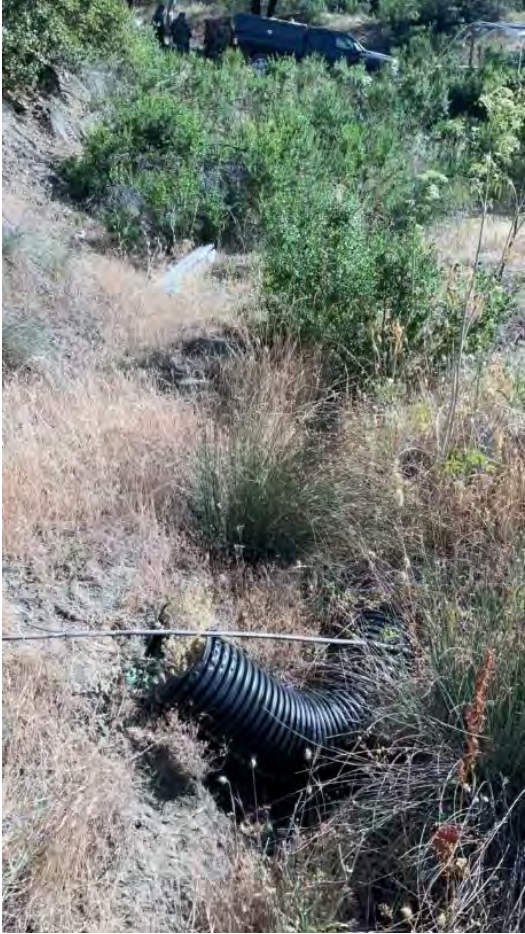
Figure 12. The road rills described at Point Location 3 connect to a drainage feature with a defunct flexipipe installed from the road edge downslope along Line Location 7. Photo is view looking upslope along feature to access driveway.
