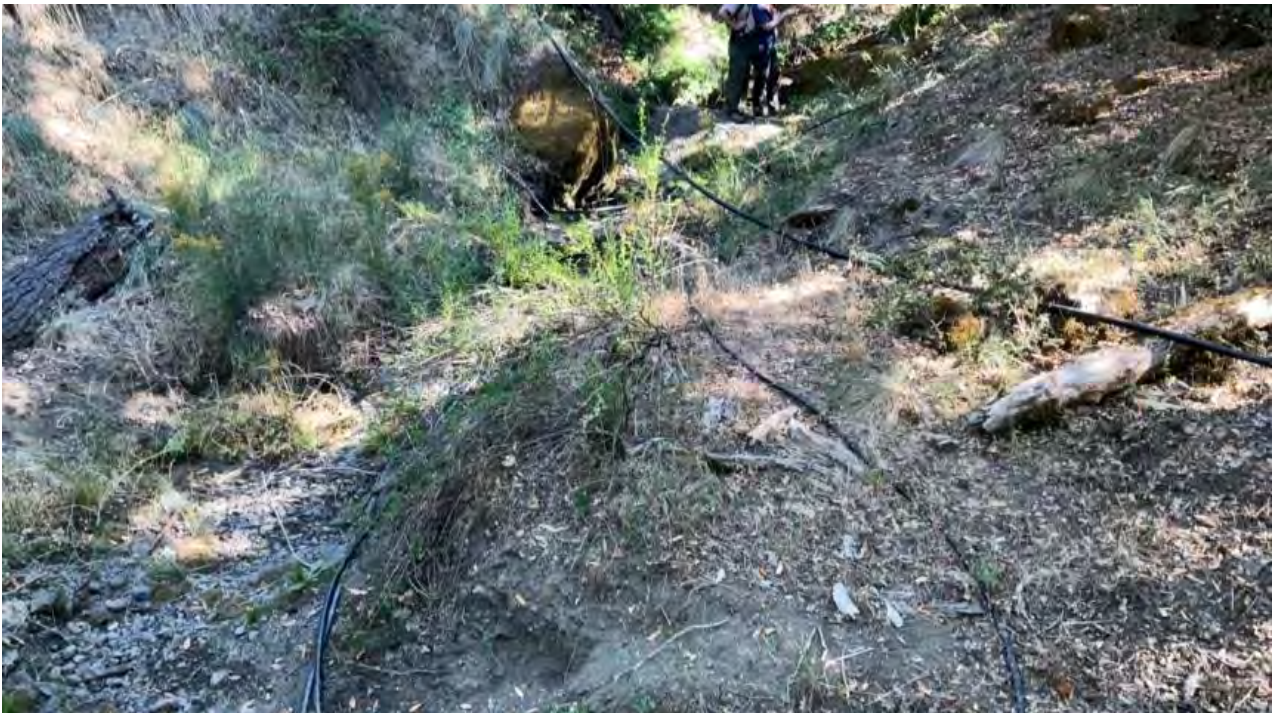
Figure 17. Just upstream of the bridge, is an in-stream excavation and berm construction at Point Location 10. Multiple lines of black plastic poly pipe are in the watercourse.
