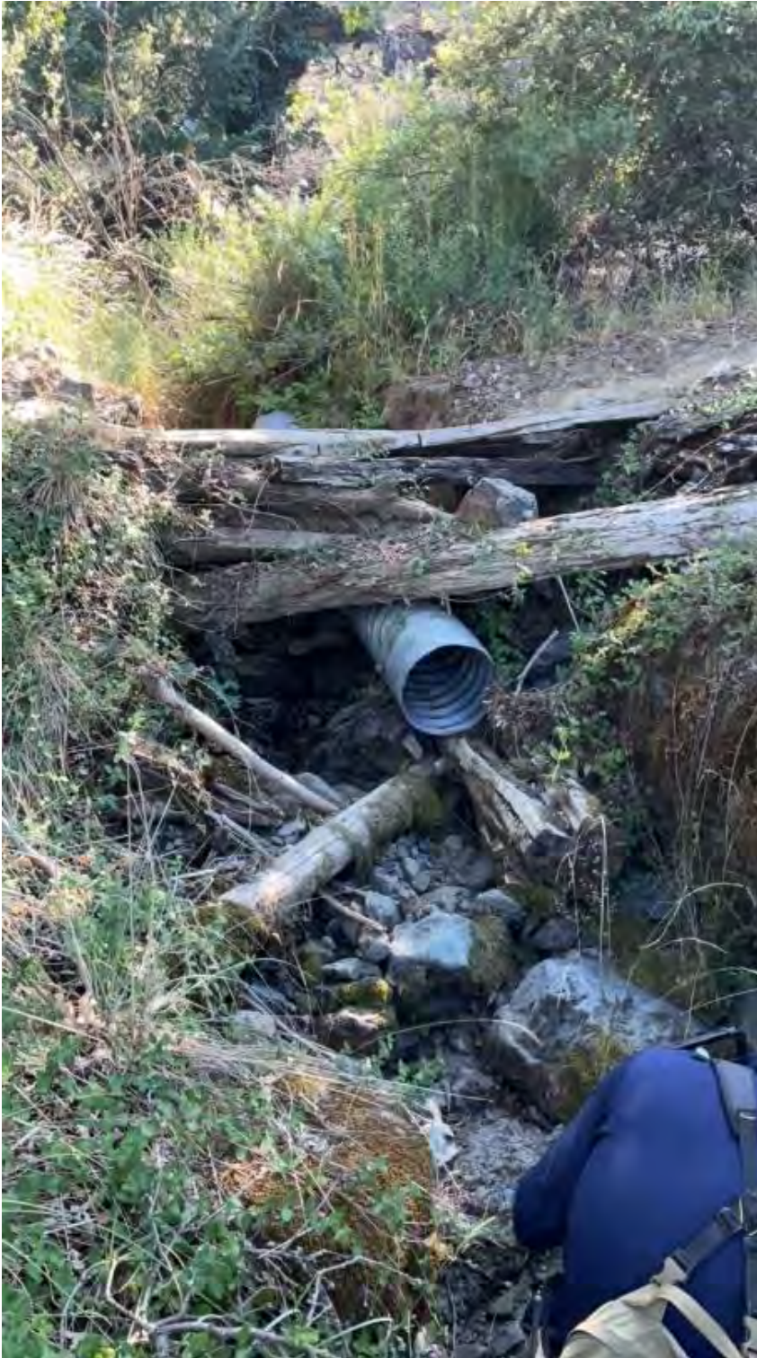
Figure 24. Stream crossing at Point Location 13 is an eroded, twelve-inch diameter, ten-foot-long corrugated metal pipe. The channel is comprised of cobble. The stream crossing was not of sufficient size to pass the 100-year flow plus debris.
