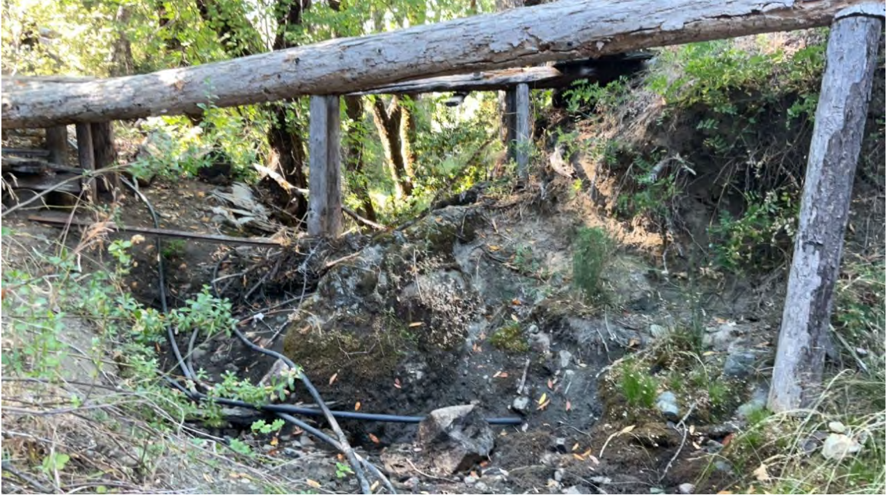
Figure 16. Bridge at Point Location 9, looking downstream from the stream bed at the piles.
