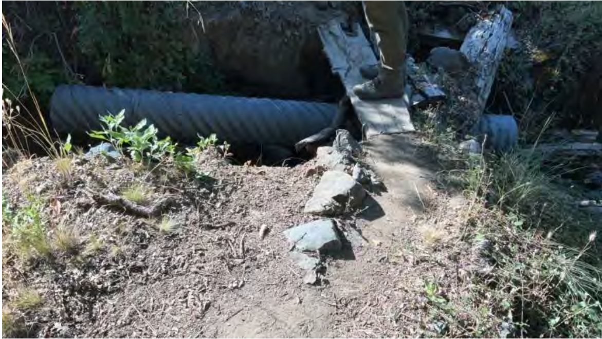
Figure 25 . The erosional void of the stream crossing fill prism at Point Location 13 is approximately five-feet deep, five-feet wide, and ten-feet long (approximately nine cubic yards of sediment delivery to a blue line stream. Immediately downstream of the crossing on the left bank is an erosion void of approximately five cubic yards of sediment delivery to a blue line stream.
