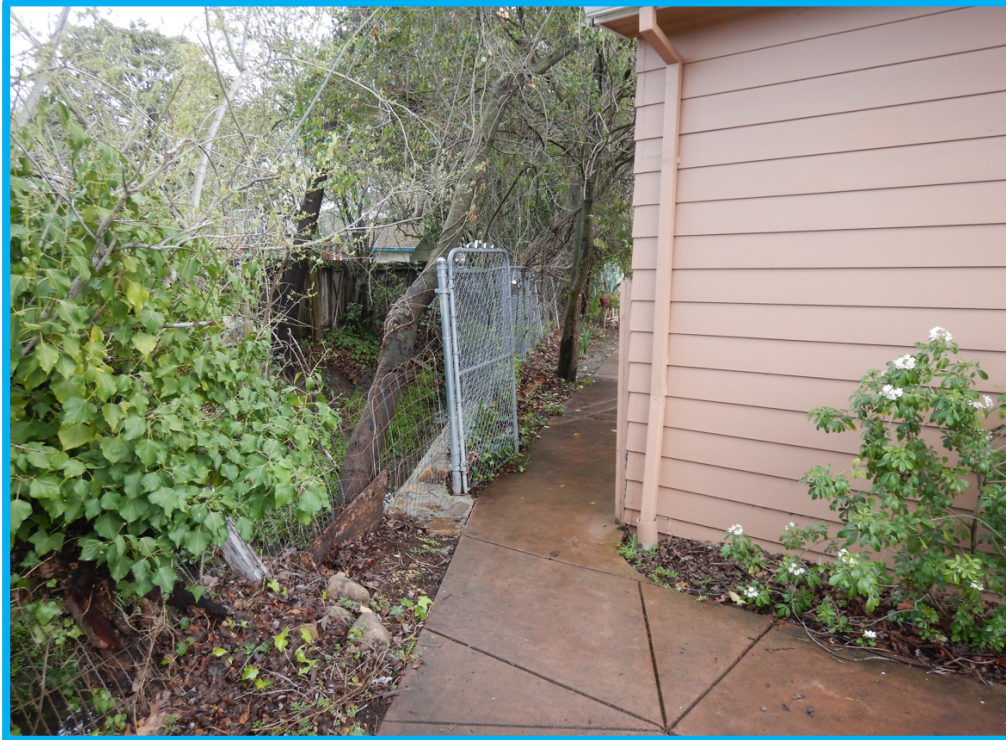
Photograph 3: Looking upstream, Mr. Olvera's garage is five feet from top-of-bank. White fence post is falling over into Poppy Creek.
