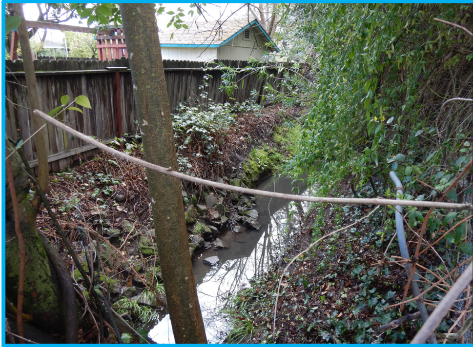
Photograph 6: looking upstream Poppy Creek of the grouted rock wall, broken concrete debris disposed on the right bank and in the active channel.
