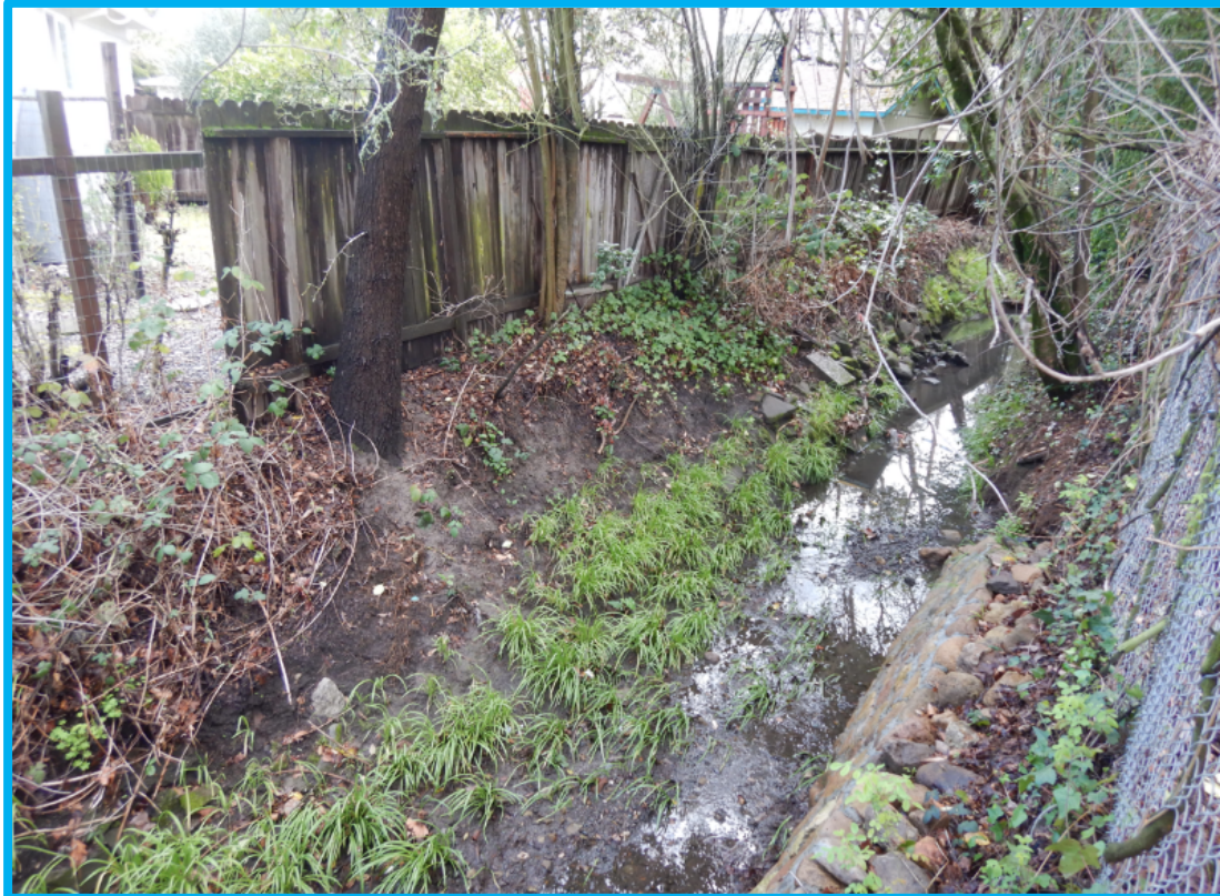
Photograph 5: Looking upstream Poppy Creek. Poppy Creek is a trapezoidal channel. High-water scour mark at bottom of wooden fence.
