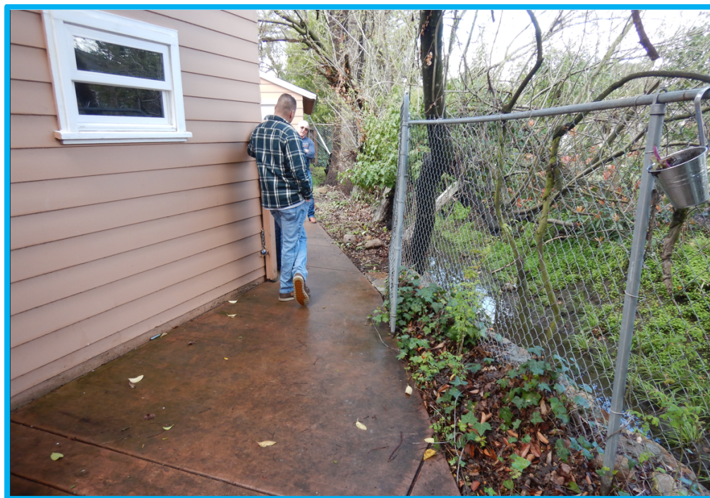
Photograph 4: Looking downstream, Mr. Olvera's garage is five feet from top-of-bank. White fence post is falling over into Poppy Creek.
