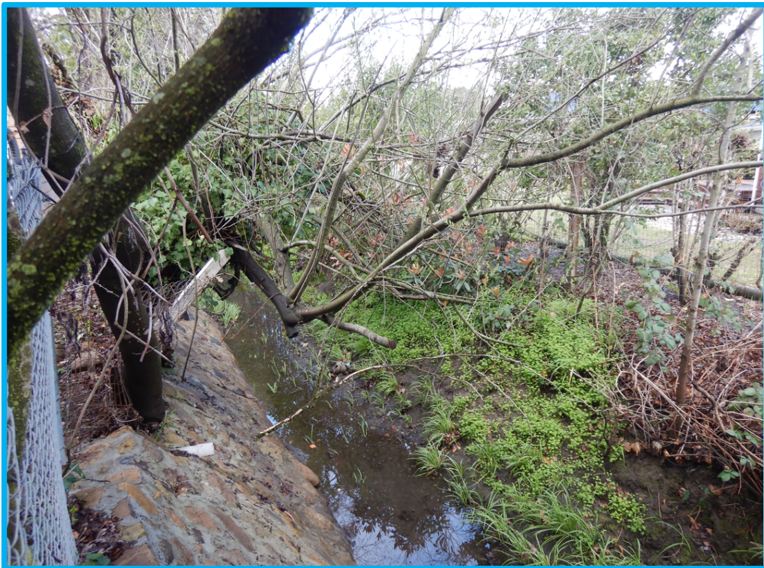
Photograph 8: Grouted rock wall placed at an estimated 65° angle and constricting the Poppy Creek channel.
